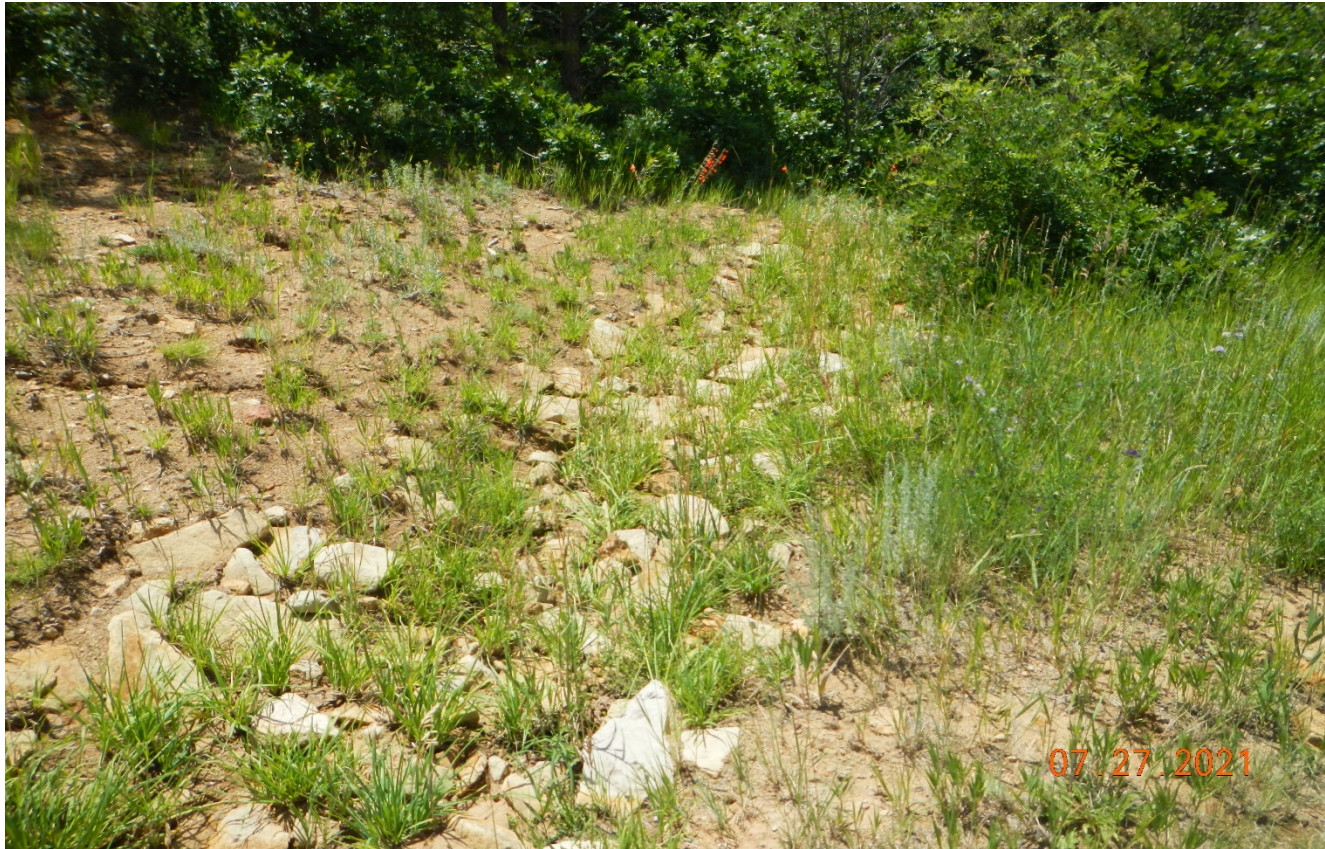
Photo 6. There is rock rip/rap installed for stormwater drainage at the south side of the location.
