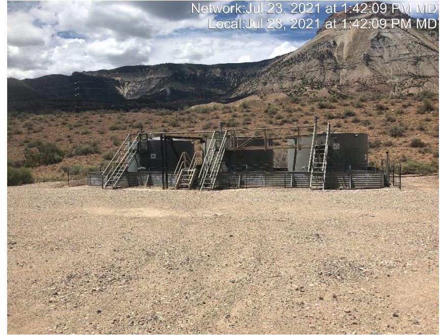
Photo #4580 No battery sign located at the tank battery.
