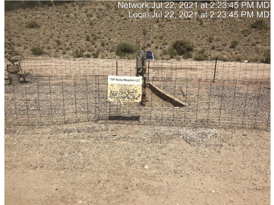
Photo #4562 Wellhead sign weathered and not legible.
