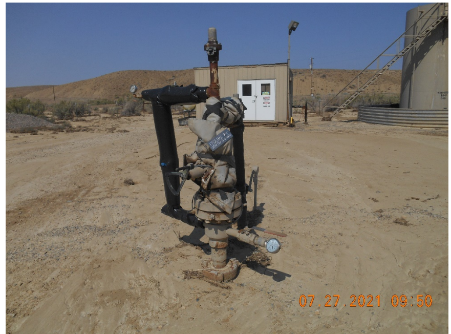
Wellhead with pump housing in background.
