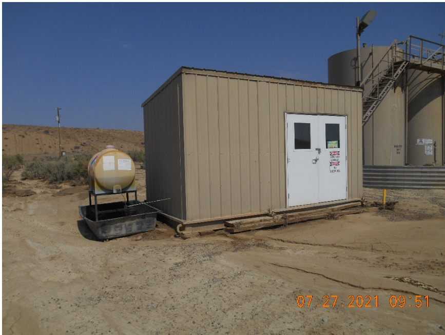
Pump housing. Labels on chemical tank illegible.
