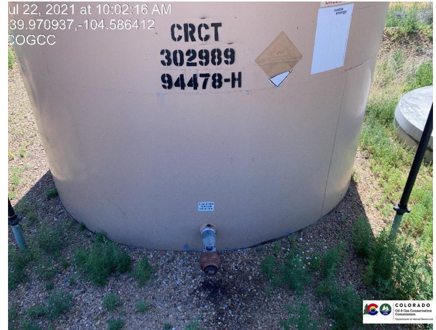
Pic 2 stained soil / placard needs replaced
