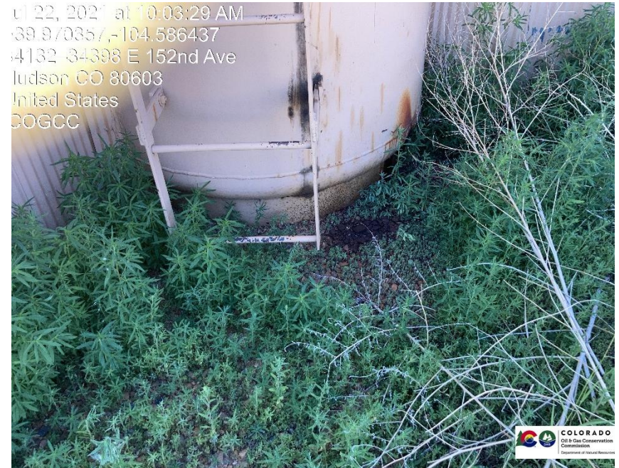
Pic 4 stained soil / mechanical issue
