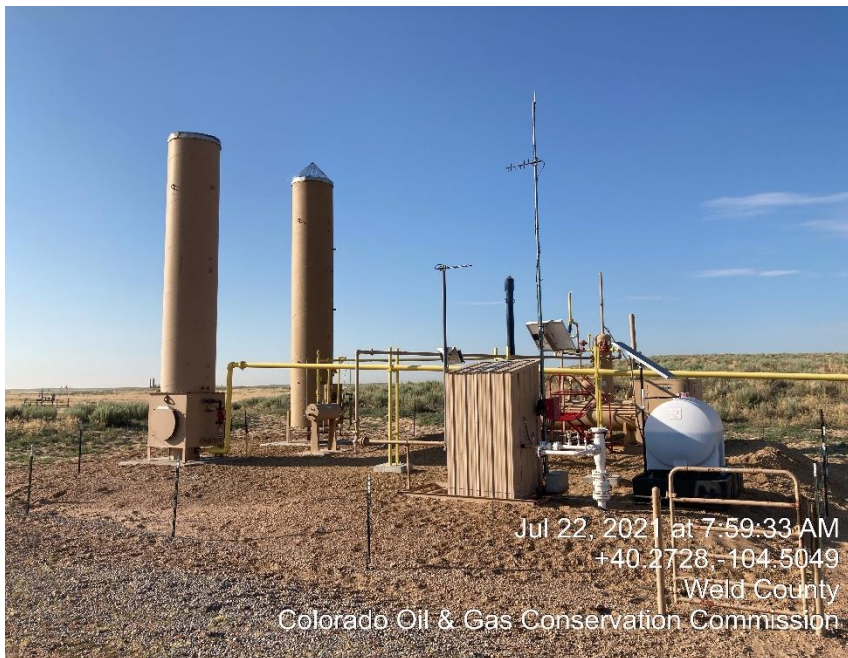
Photo #2 Production Equipment
