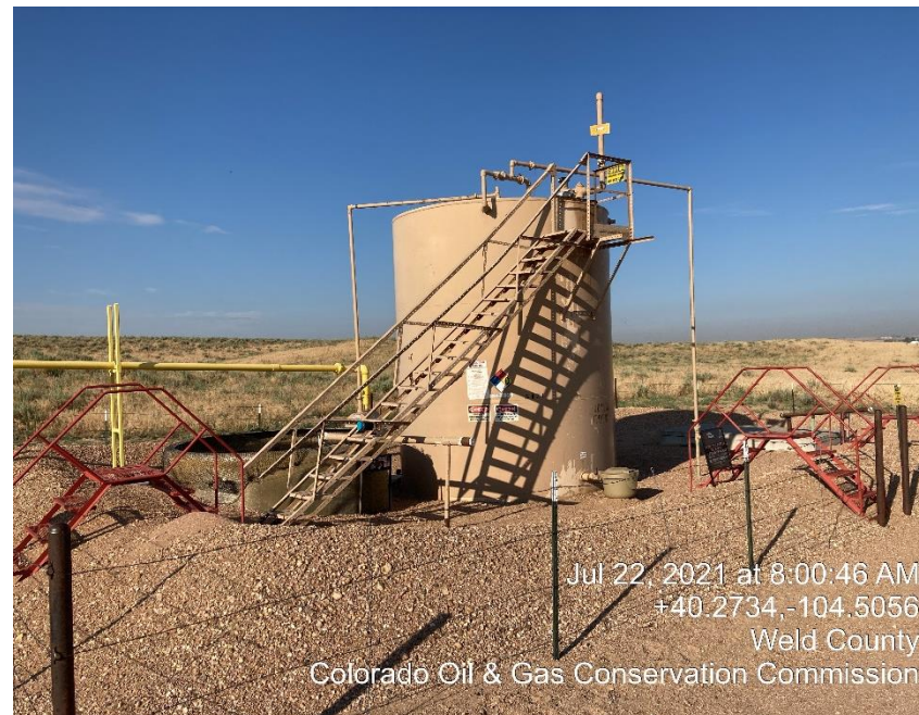
Photo #3 Tank Battery
