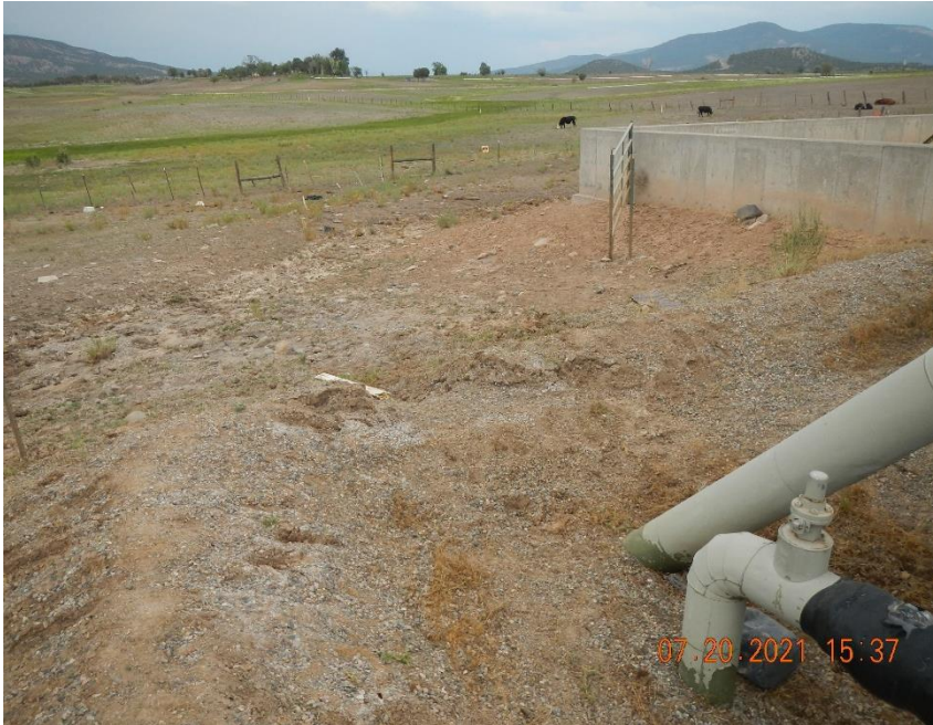
Secondary containment berm has been breached.
