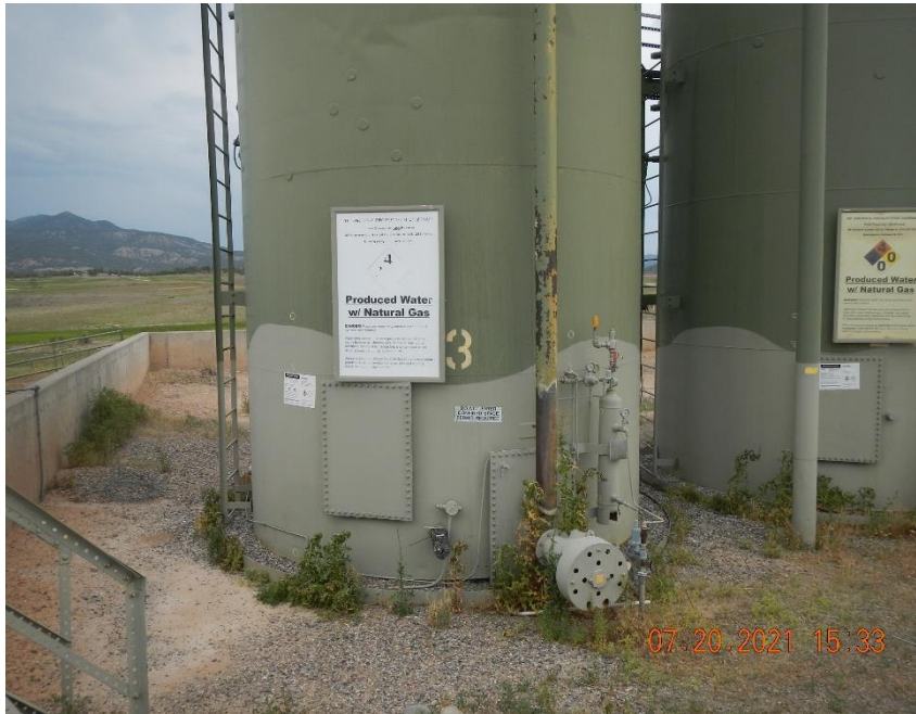
Weeds present within secondary containment area. Tank label on western AST is illegible.
