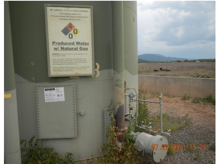
Weeds present near fired equipment.
