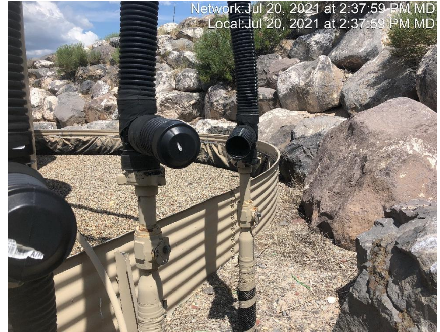
Photo #4515 Flow line heating insulation open ended and not capped.
