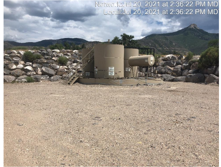
Photo #4513 No battery sign located at the tank battery.
