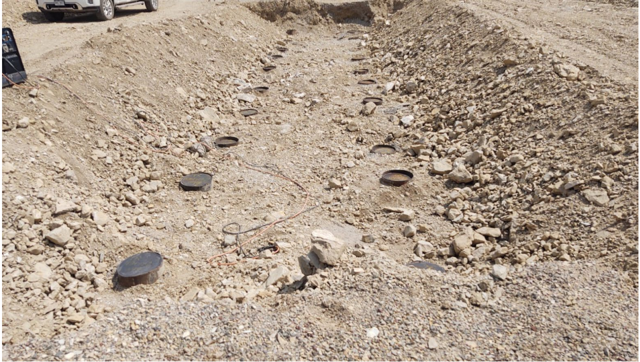
Conductors plugged on the Chevron TR 43-32-597 Well Pad on 7/14/2021
