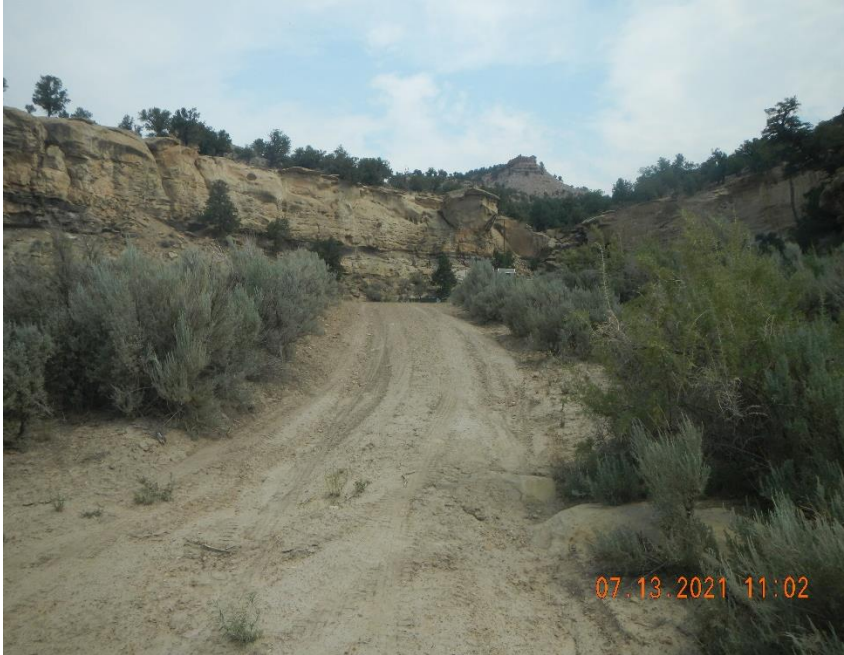
Access road is not maintained. Boulder with hole created by traffic at entrance to DTU 1056.
