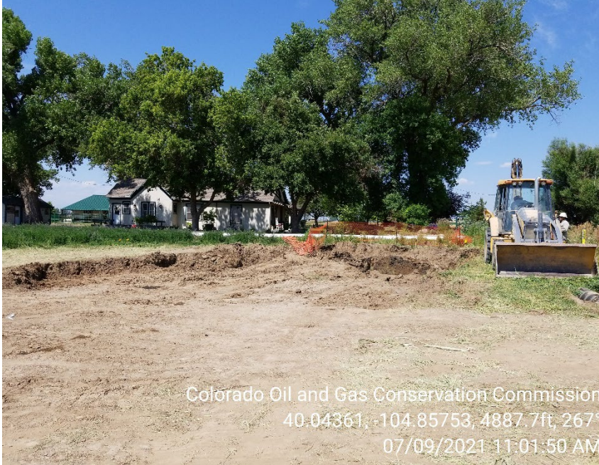
Photo 1 – Spill area 7/9. Excavation is open and surface soils surrounding excavation have been scraped.
