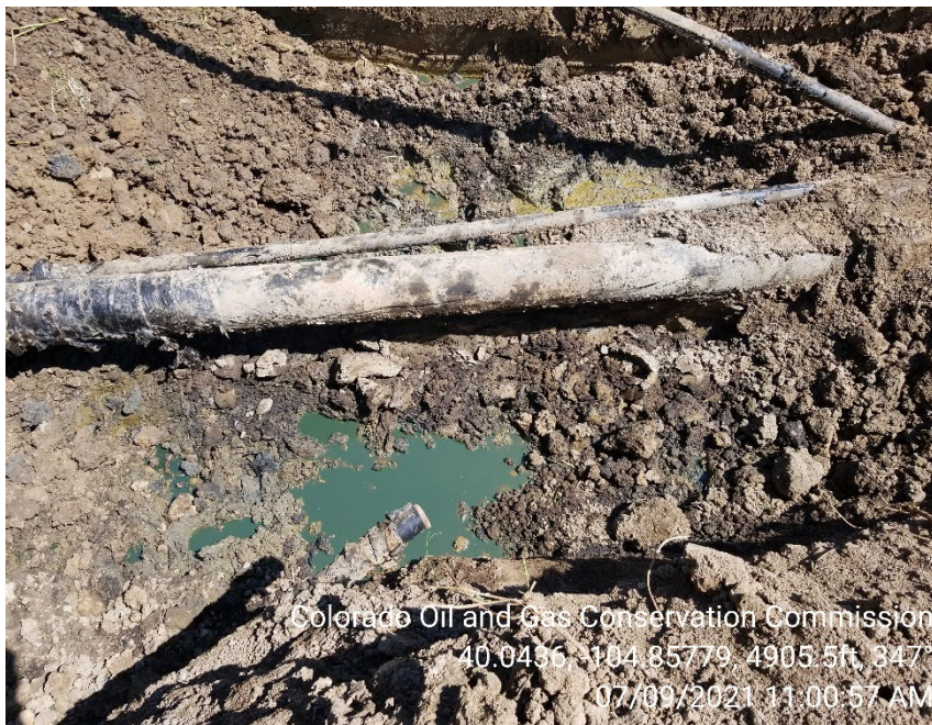
Photo 3 – Spill excavation 7/9; free product is visible in excavation.
