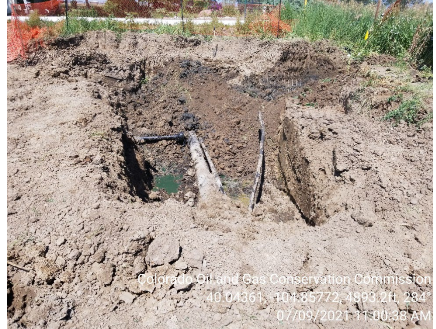
Photo 2 – Spill excavation 7/9. Impacts remain visible in-situ and free product is visible in excavation.
