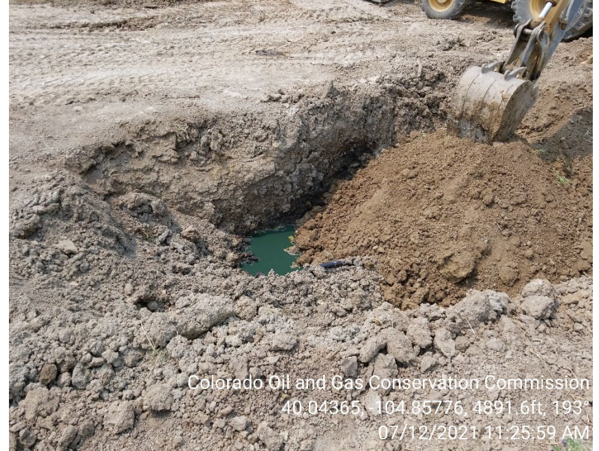
Photo 6 – Spill excavation 7/12; free product is visible in excavation and soil impacts remain in-situ.
