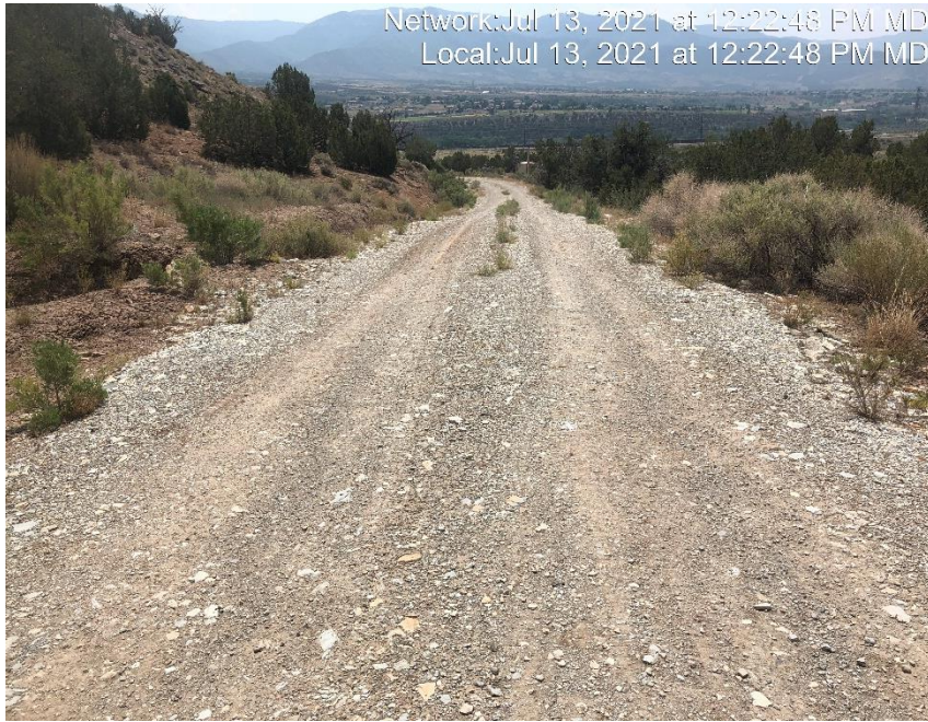
Photo #4408 No form of tracking BMP located at the entrance to location.
