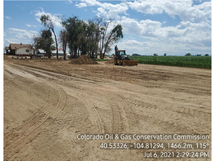
Photo 2: Location of tank battery
