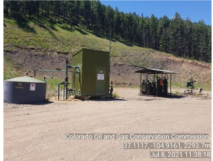
Photo 4 5-12v production equipment.
