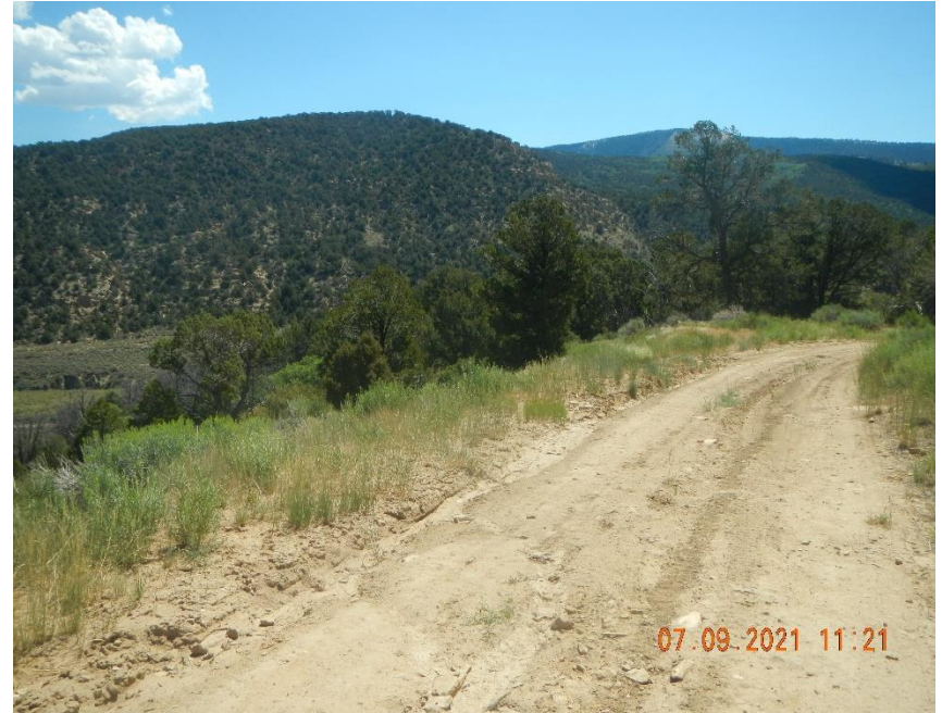
Access road and ditch need maintained.
