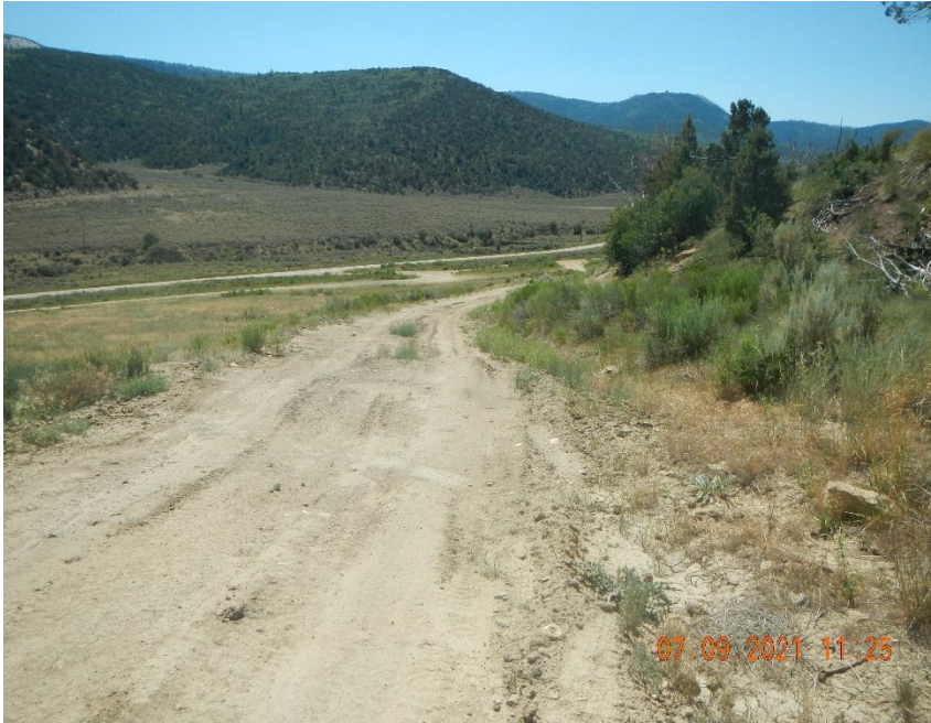
Access road and ditch need maintained.
