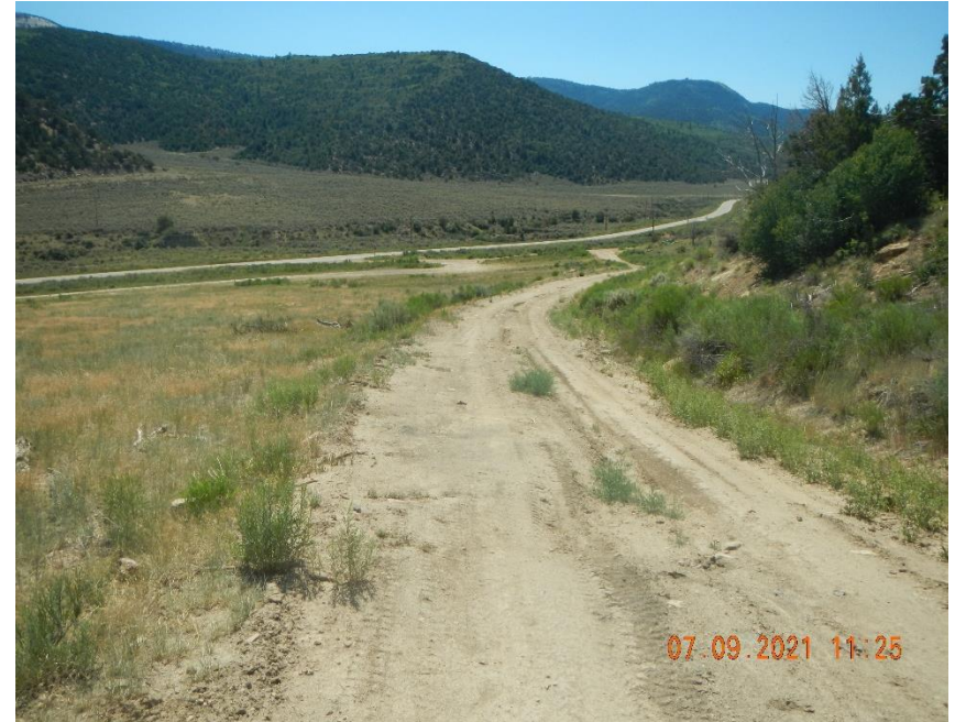
Access road and ditch need maintained.
