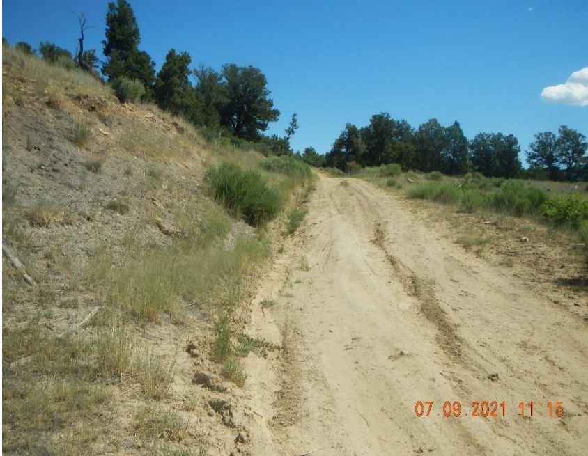
Access road and ditch need maintained.
