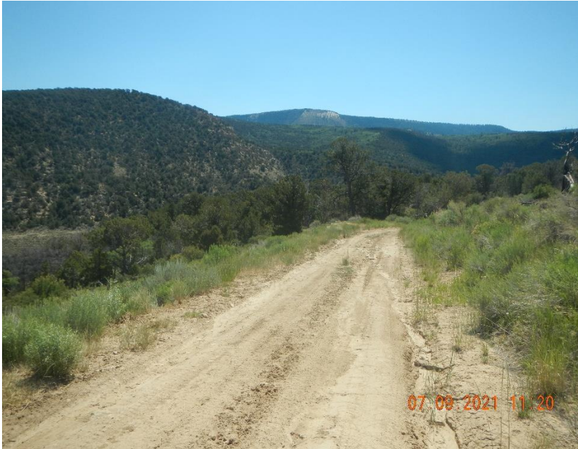
Access road and ditch need maintained.
