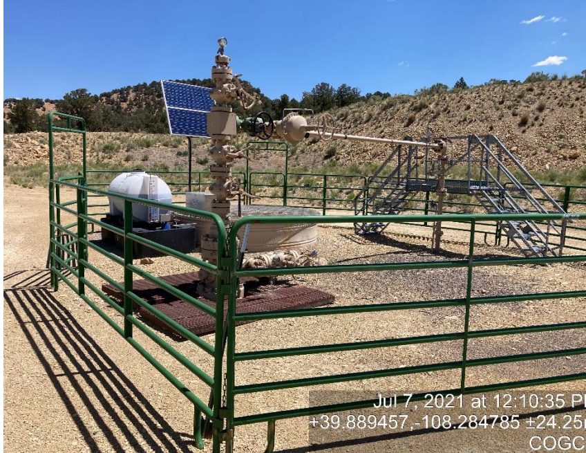
Location/ lack of wild life ramp
