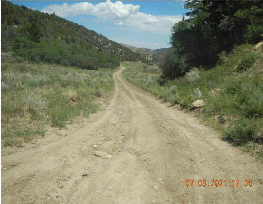
Road and road BMPs not maintained. At location Steele-B7413
