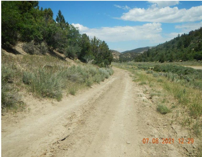
Road and road BMPs not maintained.
