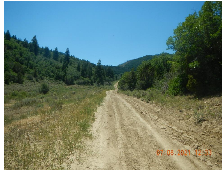
Road and road BMPs not maintained.
