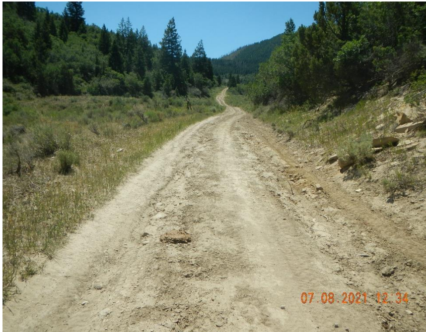
Road and road BMPs not maintained.
