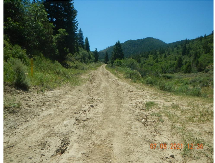
Road and road BMPs not maintained. From location Steele-B 7413 to location FOUNDATION CREEK B 7407
