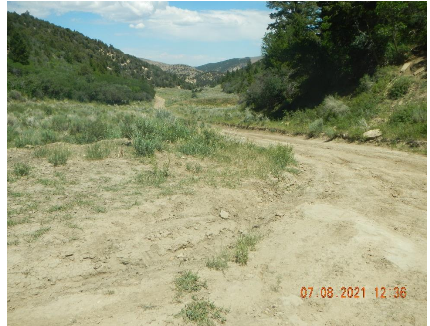
Road and road BMPs not maintained.
