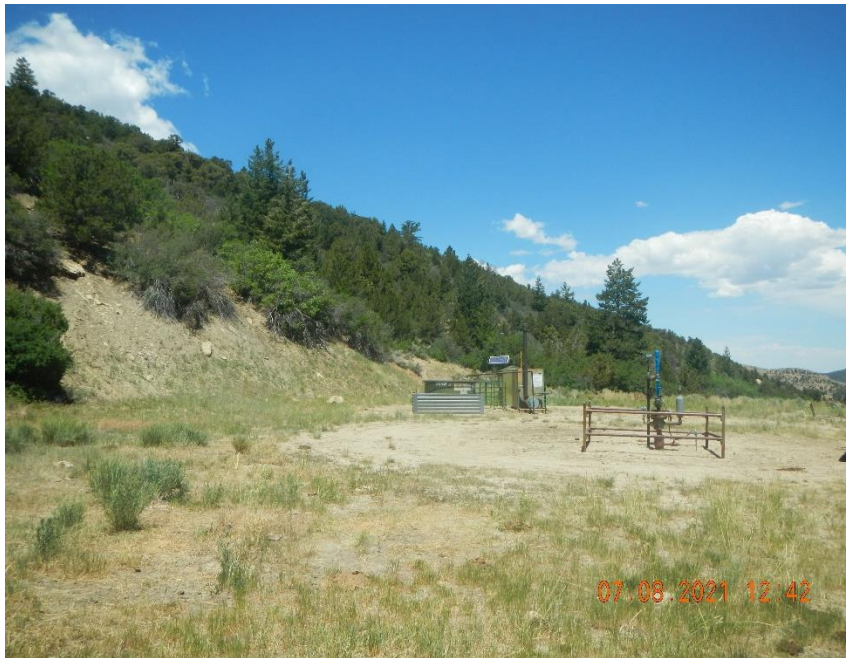
No battery sign at tank battery.
