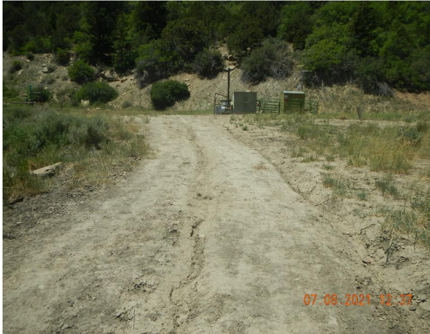
Ruts washing from location to access intersection.
