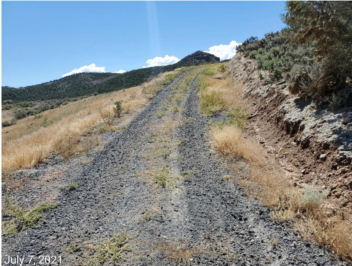
Photo 3: Photo taken from the access road facing southeast. Photo shows access road has not been reclaimed in accordance with 1004 Rules and corrective actions.
