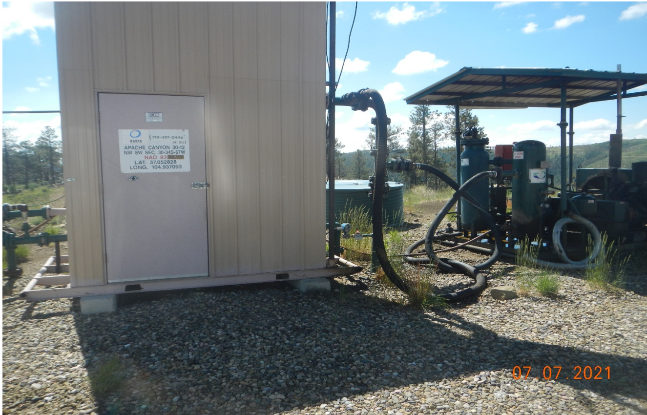
Photo 3. Well sign posted at meter shed.
