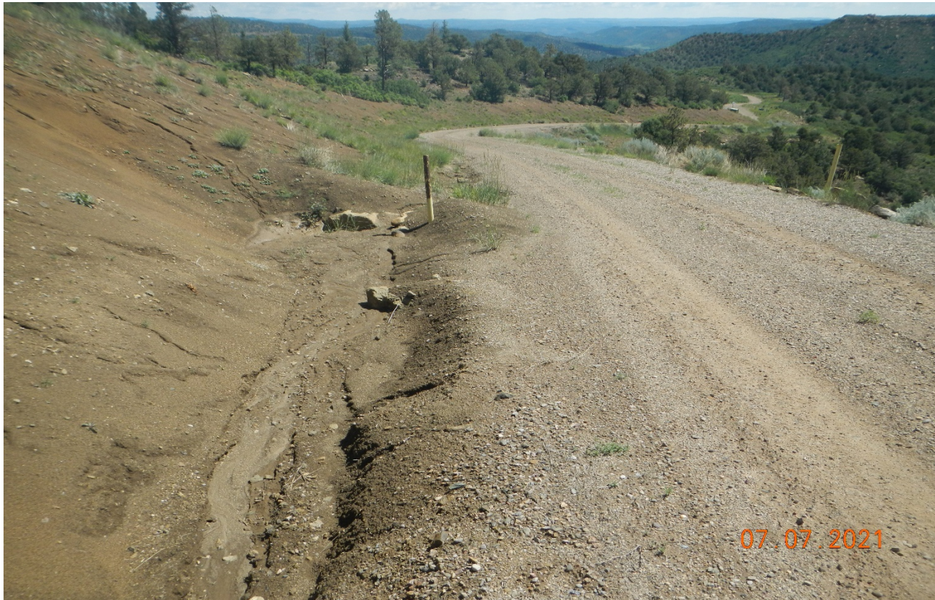
Photo 2. There are multiple culverts along the road that are filled in with sediment.
