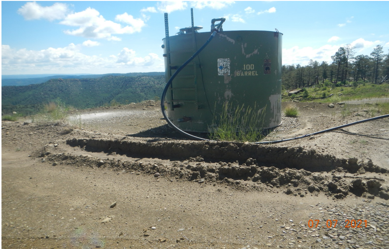
Photo 5. The berm around the tank is insufficient to contain a spill.
