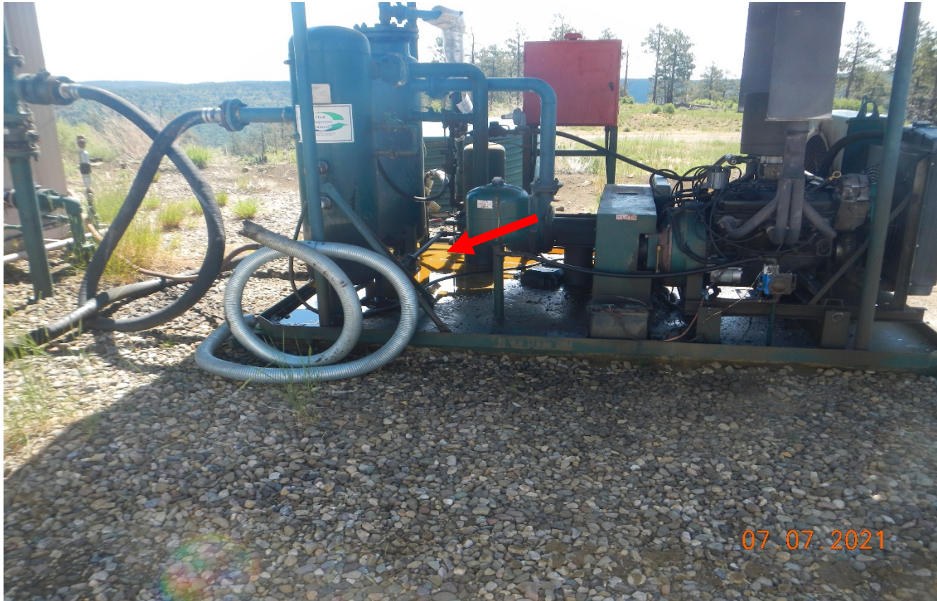
Photo 4. There is oil fluid in the engine skid shown at red arrow.
