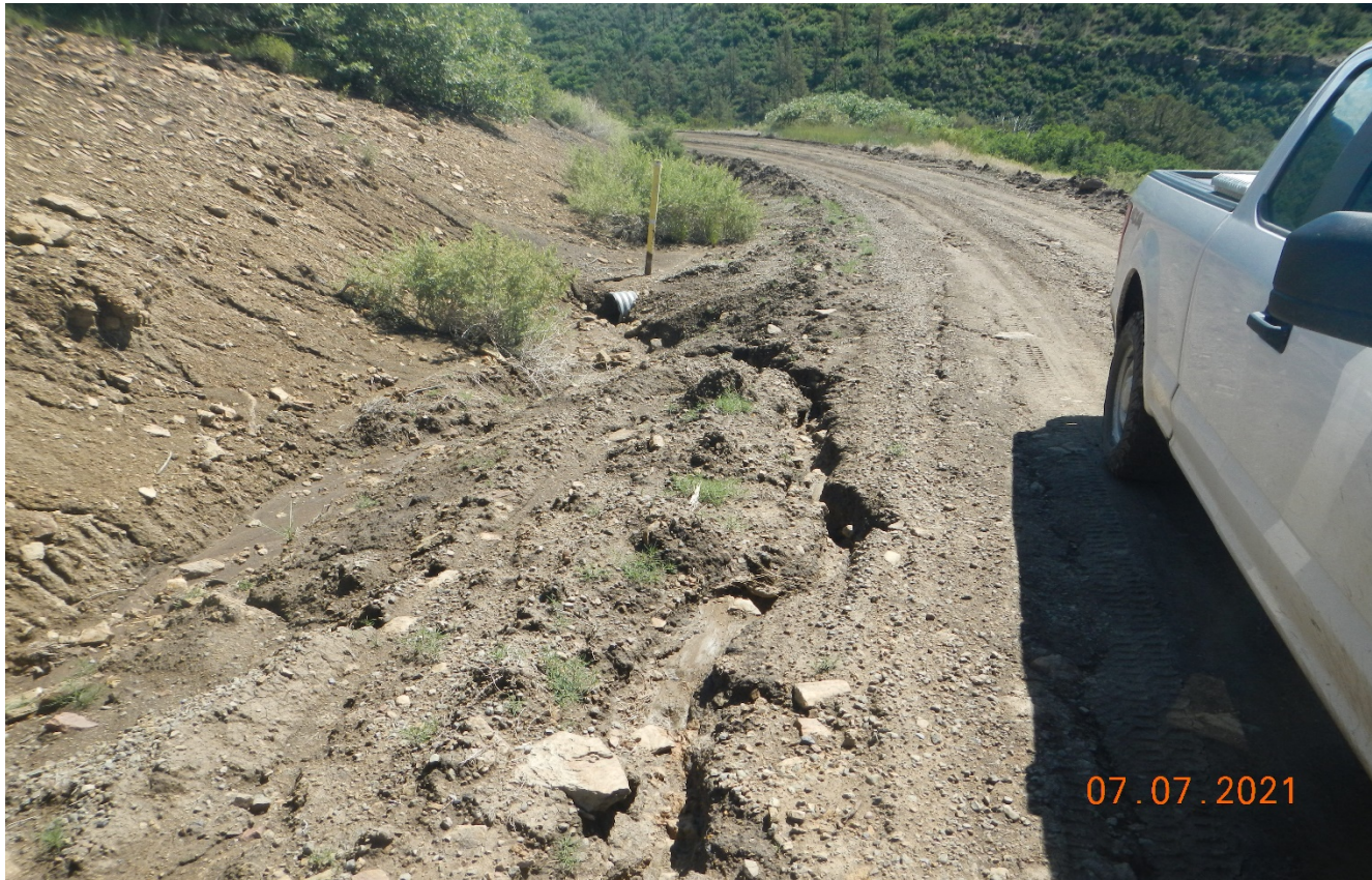
Photo 2. Erosion is occurring along the road which is not stabilized.
