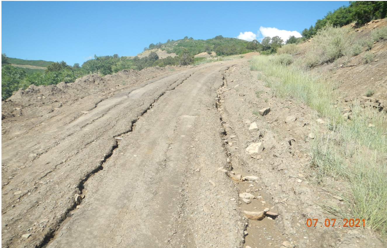
Photo 3. Erosion is occurring along the road which is not stabilized.
