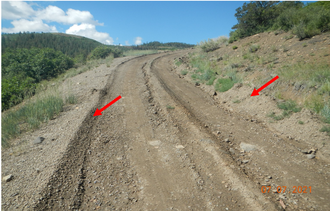
Photo 1. Facing southwest along the access road. There is erosion occurring along the road and gravel has been graded off the road shown at red arrow.
