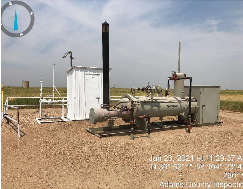
Photo #3 meter & separator.
