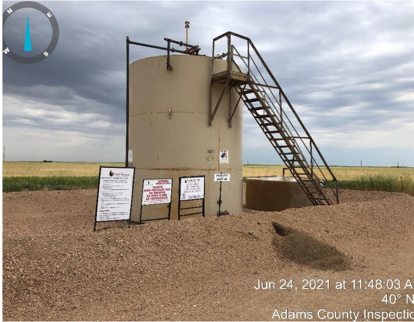
Photo #1 crude tank.
