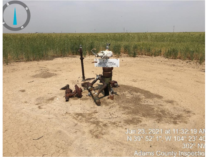
Photo #4 well head.
