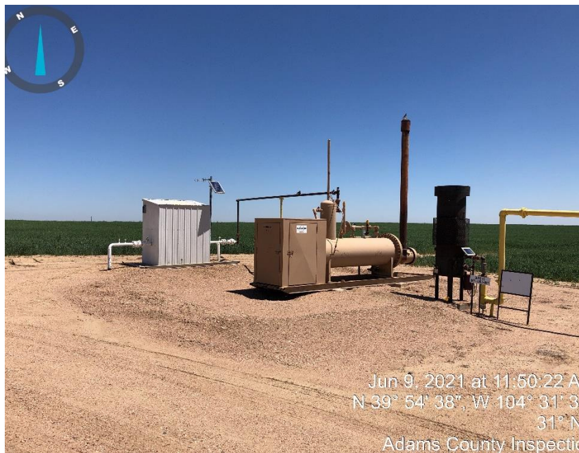
Photo #2 Meter, Separator, ECD.
