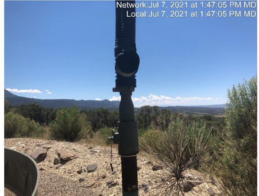
Photo #4345 Flow line heating insulation open ended and not capped.
