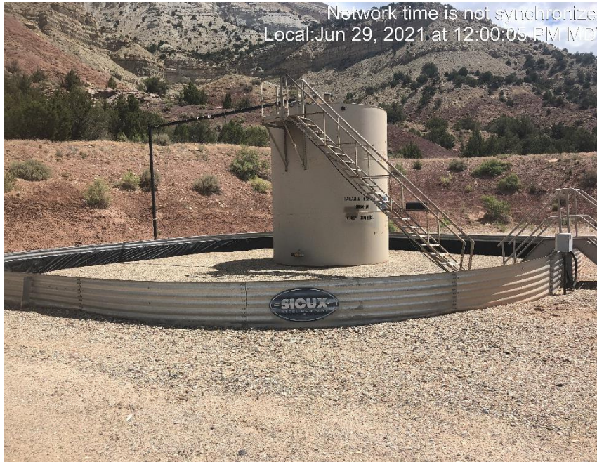
Photo #4218 No battery sign located at the tank battery.
