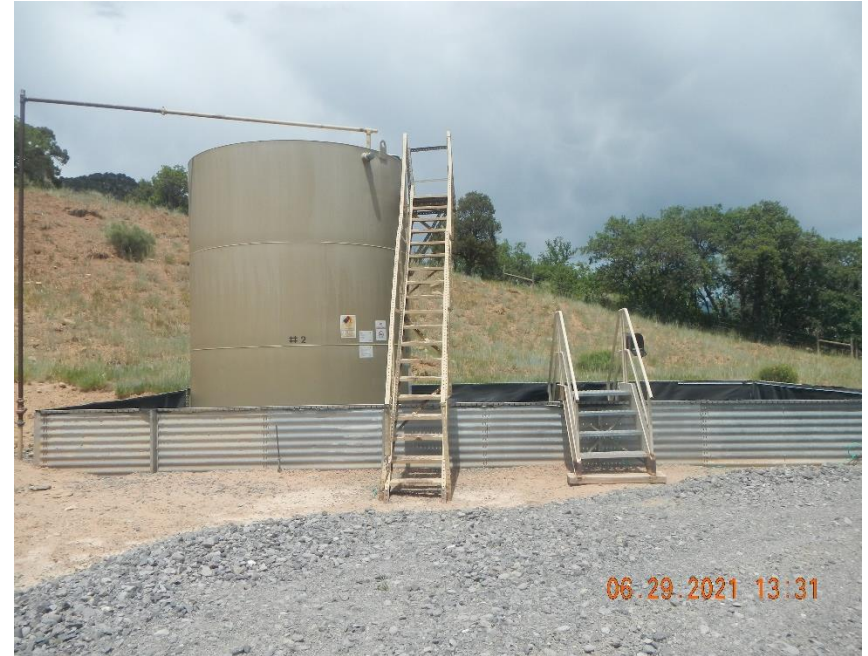
No battery sign at tank battery.
