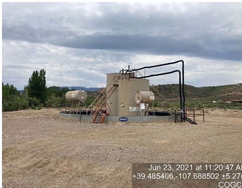
Location/lack of battery signage
