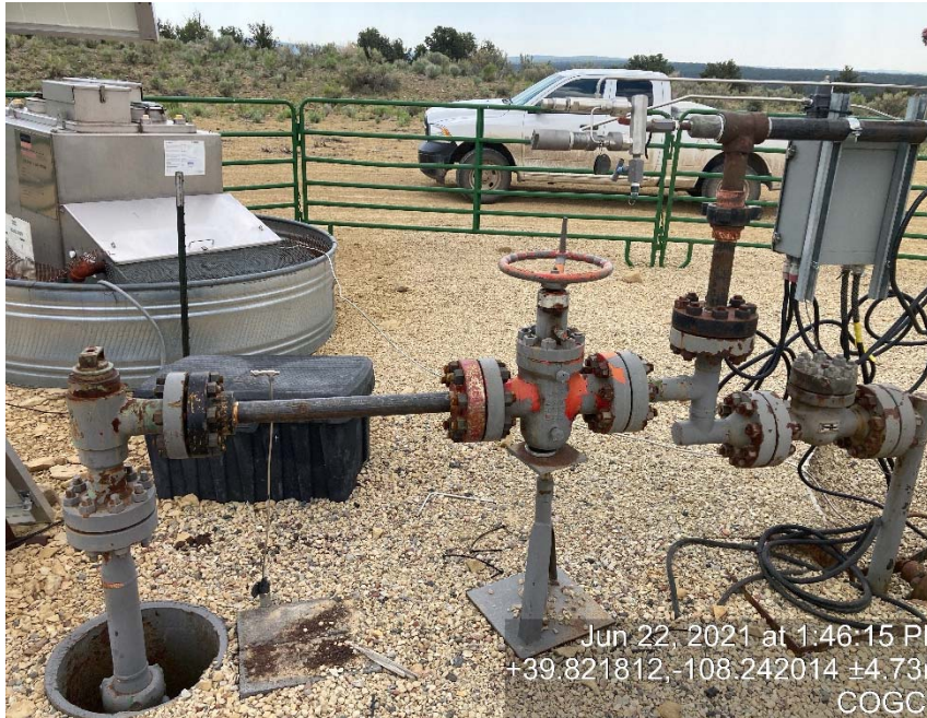
Lack of well head signage
