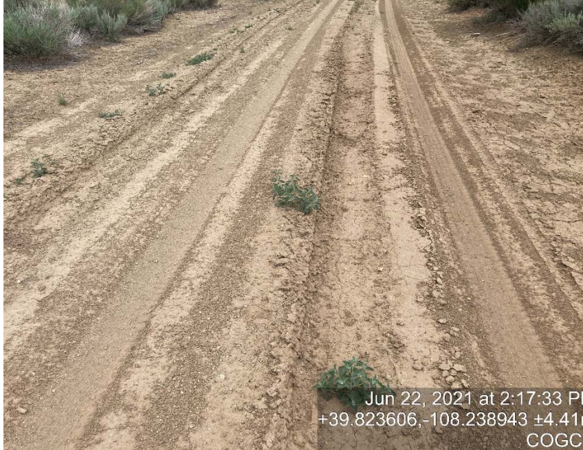
Lack of stabilization/compaction
