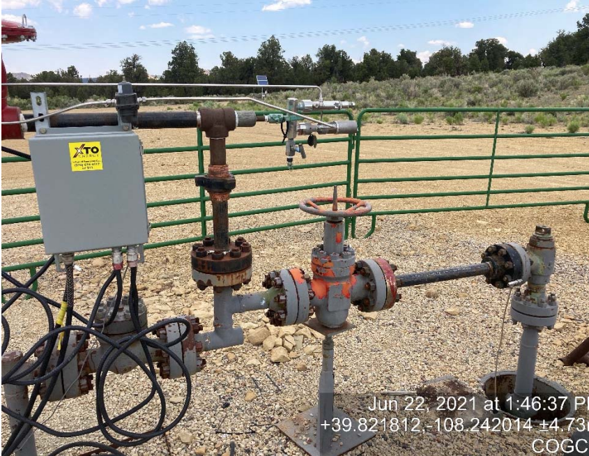
Lack of well head signage
