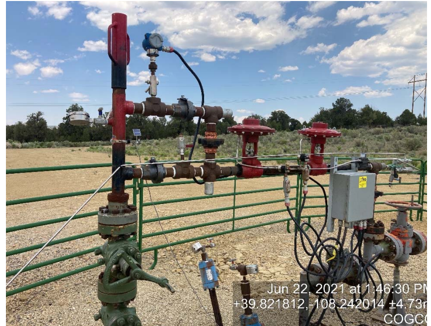
Lack of well head signage
