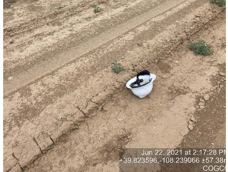
Lack of stabilization/compaction
