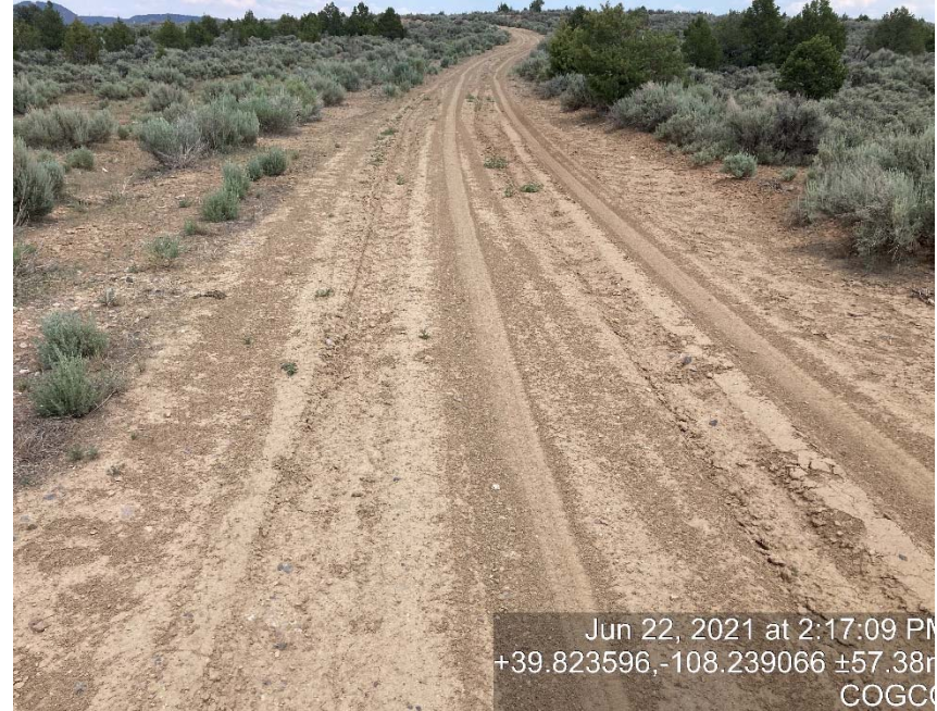
Lack of stabilization/compaction
