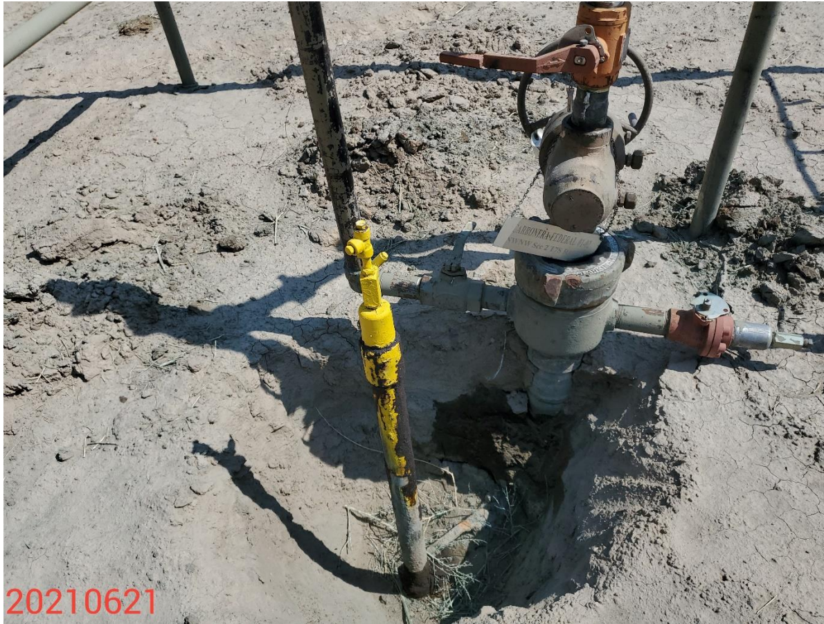
Photo 7: Photo taken from the wellhead; photo shows stained soils observed at base of well and riser; integrity concerns evident.
