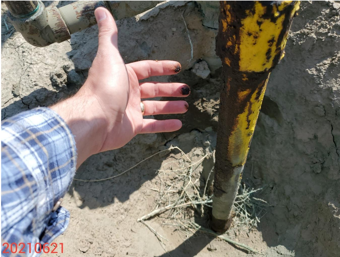
Photo 8: Continued from photo 7. Photo shows integrity and leaking concerns are evident.
