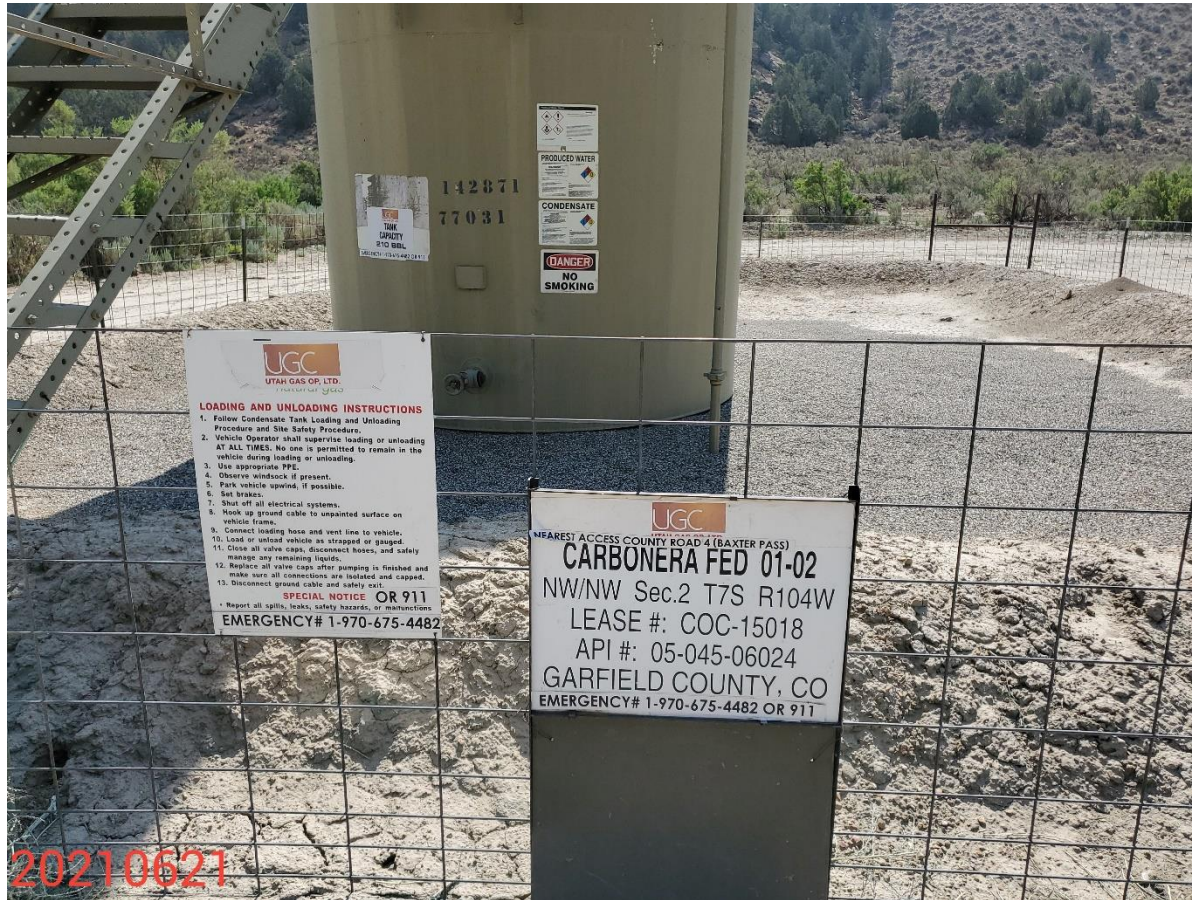
Photo 5: Photo of signage at battery facility.
