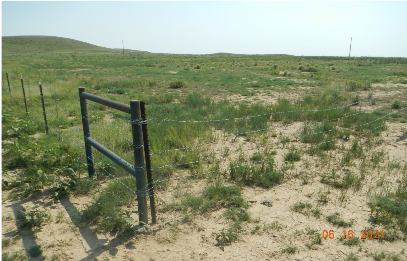
Photo 1. Facing northeast toward the location. The fence around the location is in good condition.
