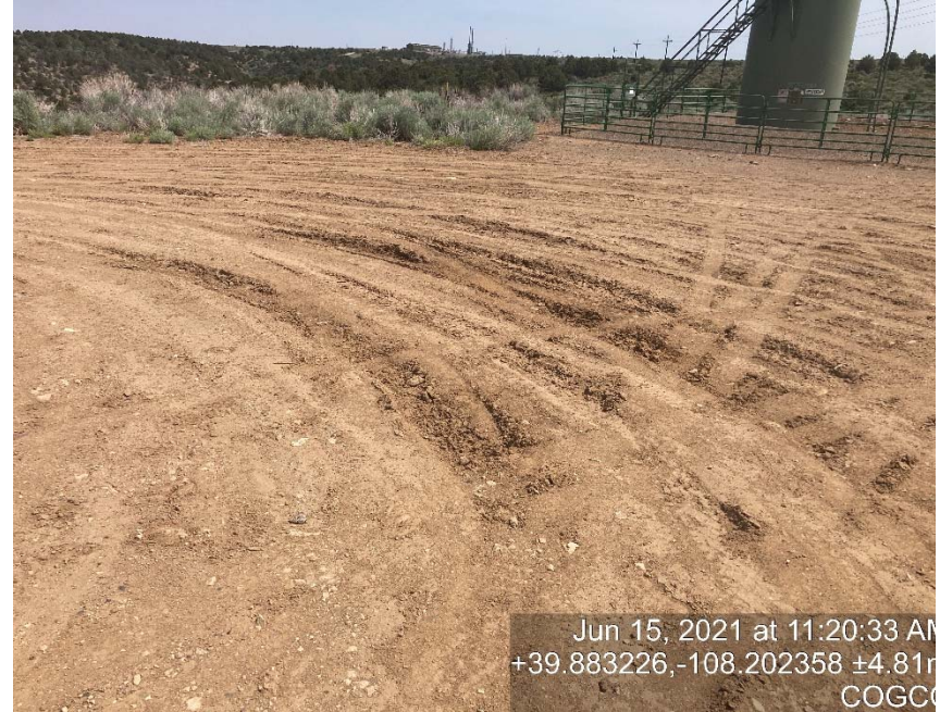
Lack of stabilization/compaction
