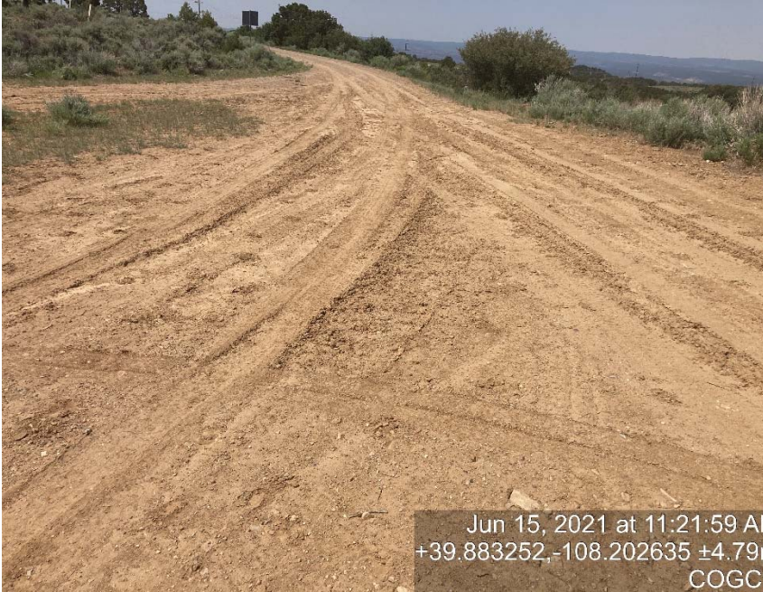
Lack of stabilization/compaction
