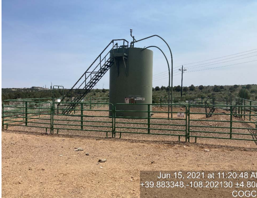
location/lack of battery signage
