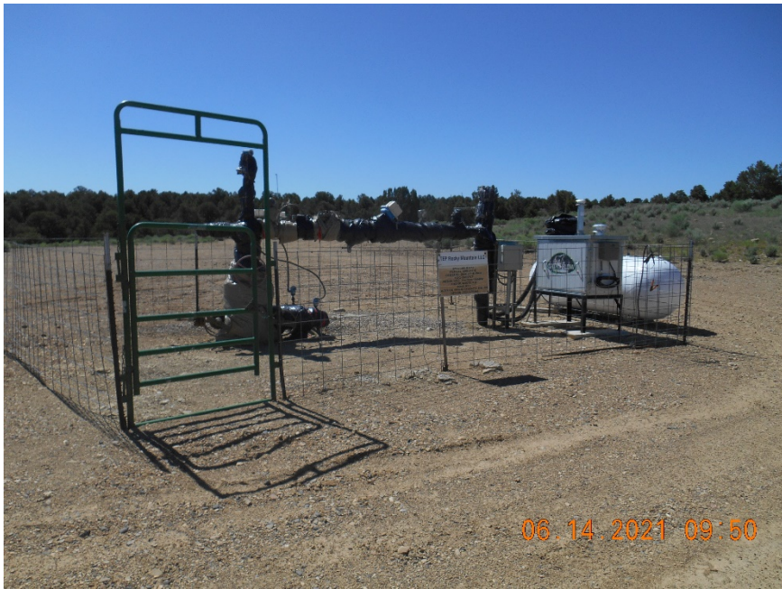
Injection wellhead & line heater
