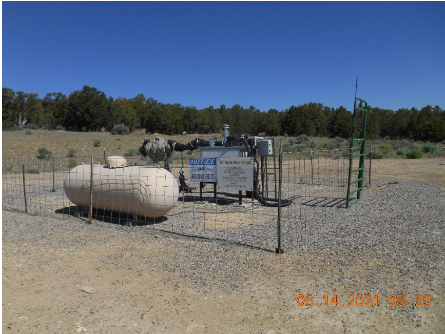
Injection wellhead & line heater
