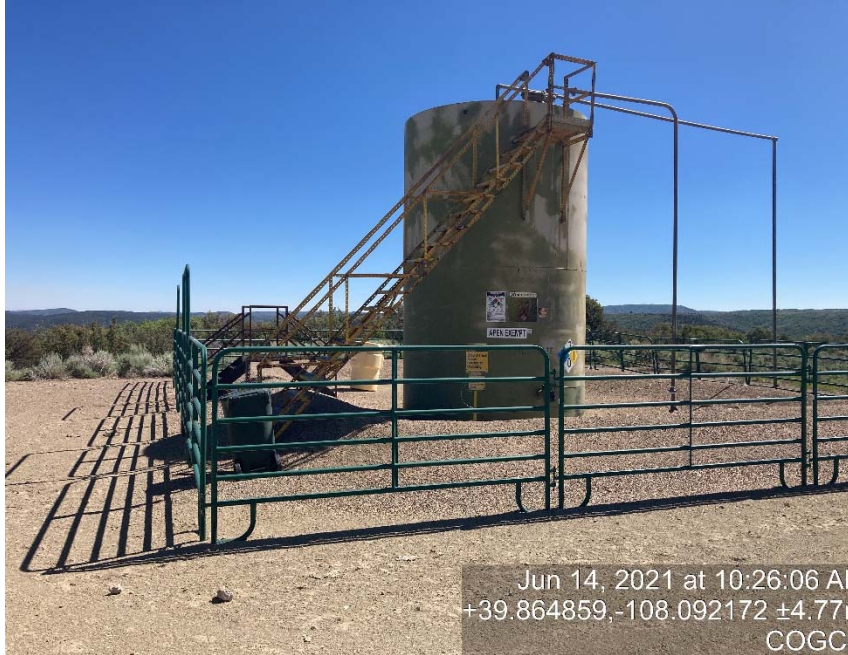
Location/Lack of battery signage
