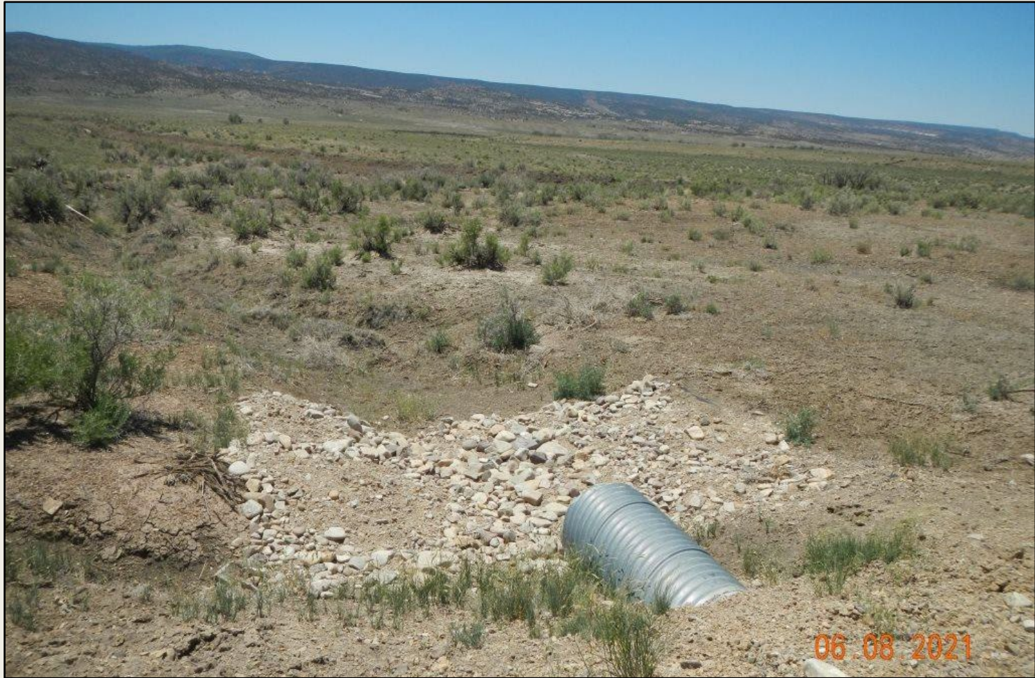
Photo 2. View of stabilization measures installed at culvert outlet along the access road in response to 2020 corrective actions.
