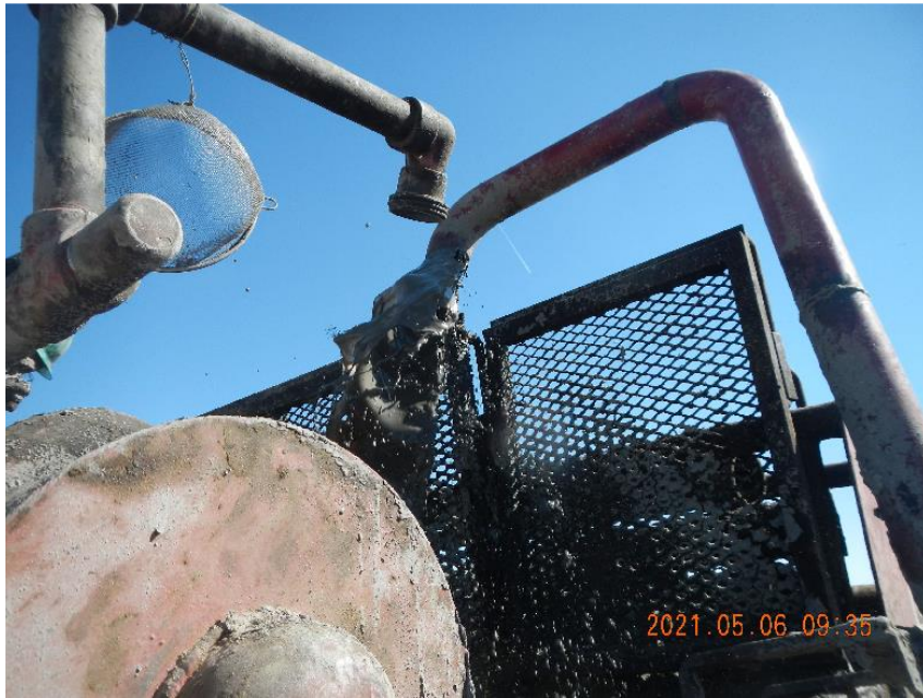
Photo 15: View of cement to the surface. Well cement work is now complete.
