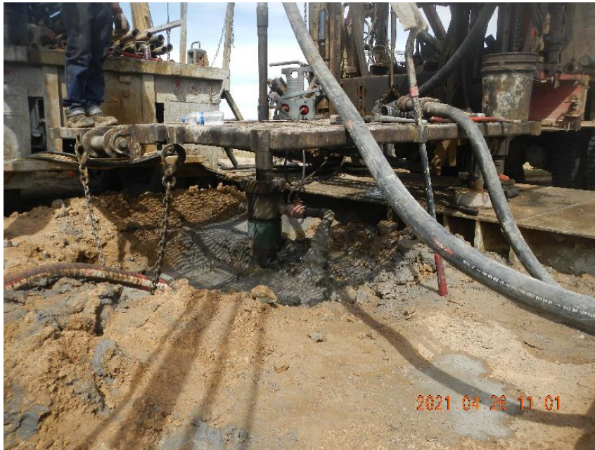
Photo 5: View of cementing work as cement was pumped to set sleeve that was run into the surface casing.
