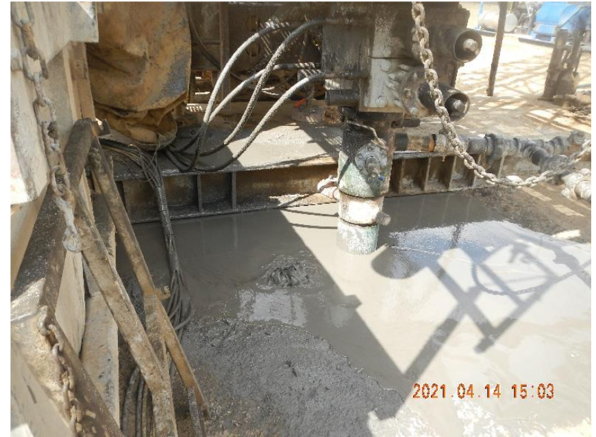
Photo 4: Fluid coming to the surface outside casing. Hole in surface casing required sleeve to be run to repair hole and continue to work down hole for cement plugs.
