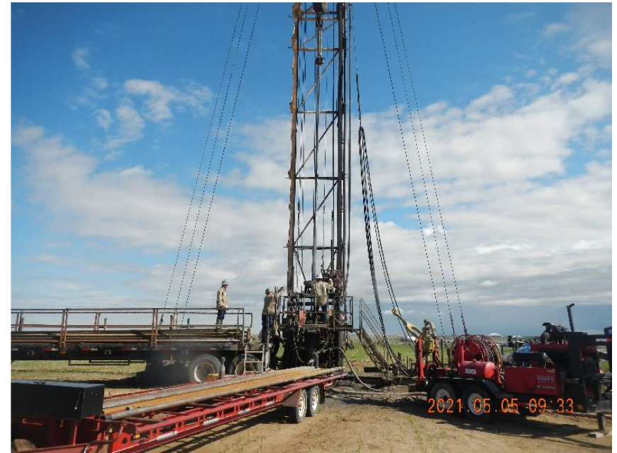
Photo 10: Rig crew tripping work string into well to tag previously pumped cement plug.
