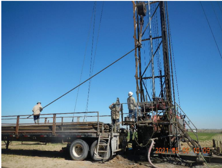
Photo 13: View of rig crew pulling and laying down work string after tagging cement plug #2.
