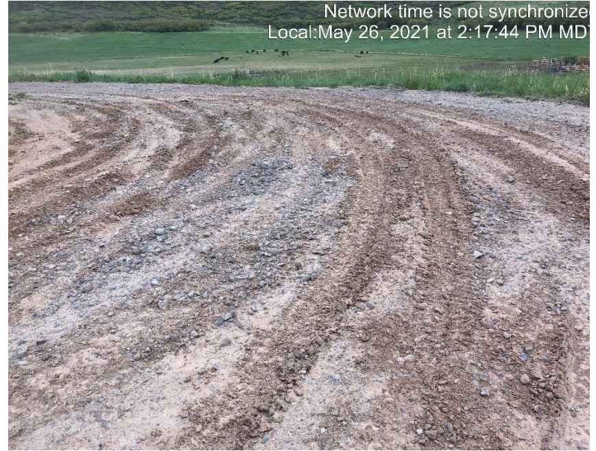
Photo #3951 Location lacks stabilization.
