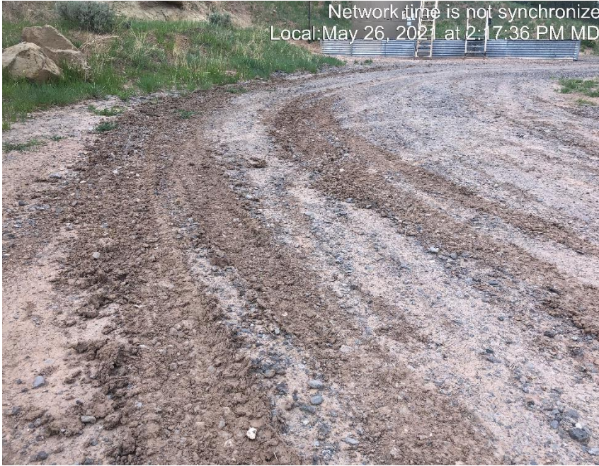
Photo #3950 Location lacks stabilization.
