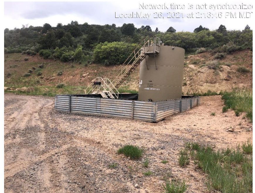
Photo #3949 No battery sign located at the tank battery.
