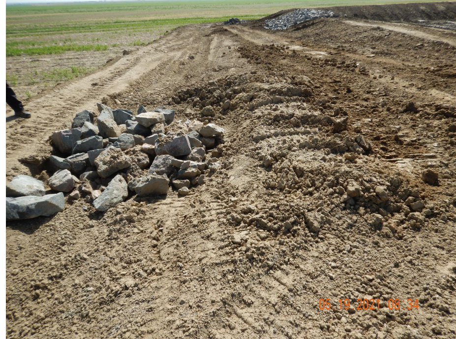
Photo 6. Photo taken from the northeastern location, facing East. Photo illustrates a check dam that is in need of further construction.
