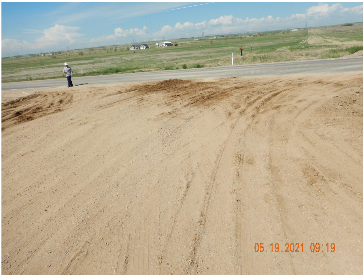
Photo 1. Photo taken from the entrance of location, facing West. Photo illustrates the major vehicle tracking device BMP has still not been installed.
