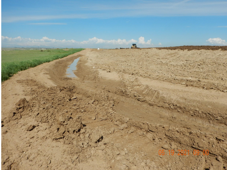
Photo 11. Photo taken from the southeastern location, facing West. Photo illustrates ponding in the ditch which is not being directed to the detention pond.
