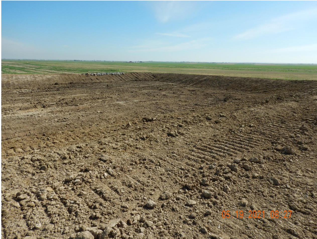
Photo 4. Photo taken from the northeastern location, facing Northeast. Photo illustrates the detention pond has been installed.
