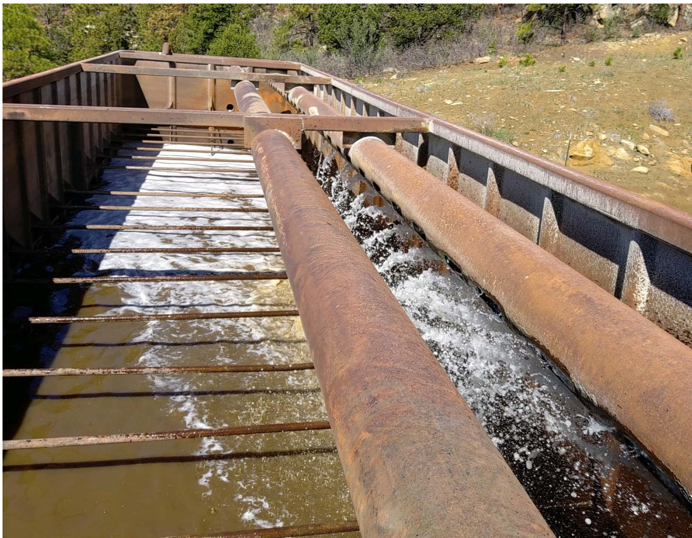
Fluid flows up hole and into open top tank.
