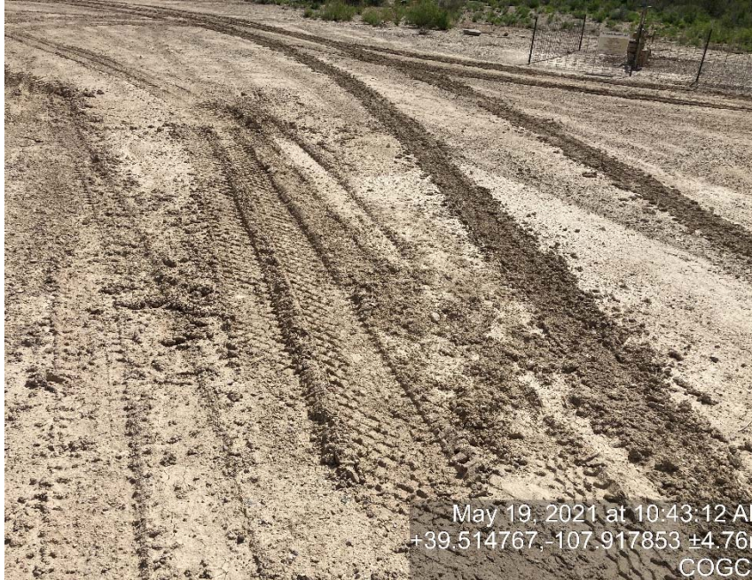
Lack of stabilization/compaction
