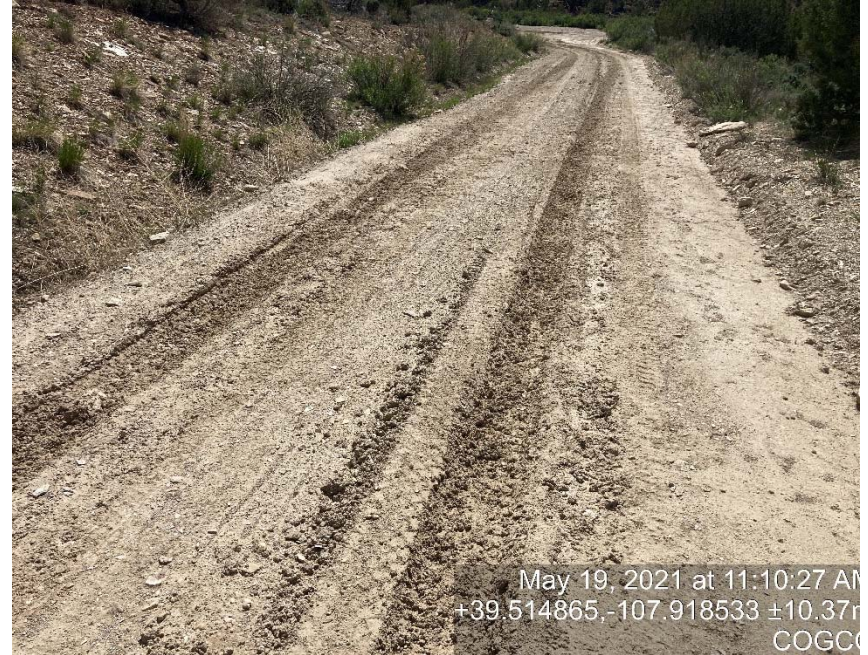
Lack of stabilization/compaction
