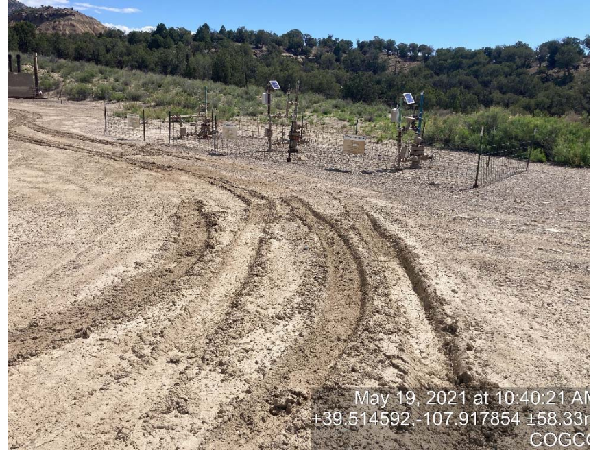
location and Lack of stabilization/compaction
