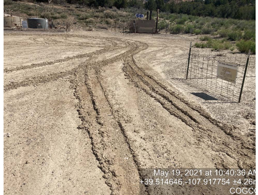
Lack of stabilization/compaction
