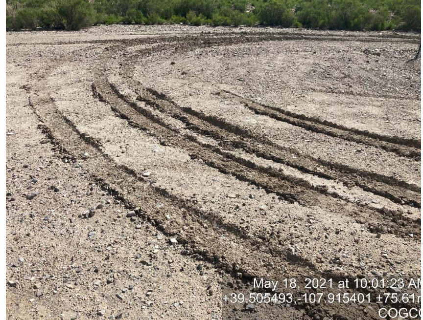
Lack of stabilization/compaction
