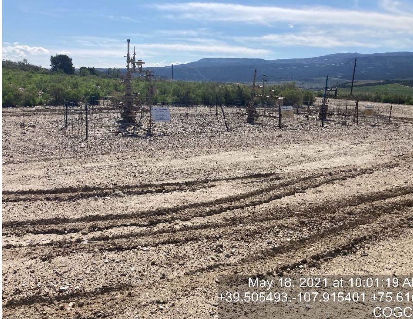
Location and Lack of stabilization/compaction
