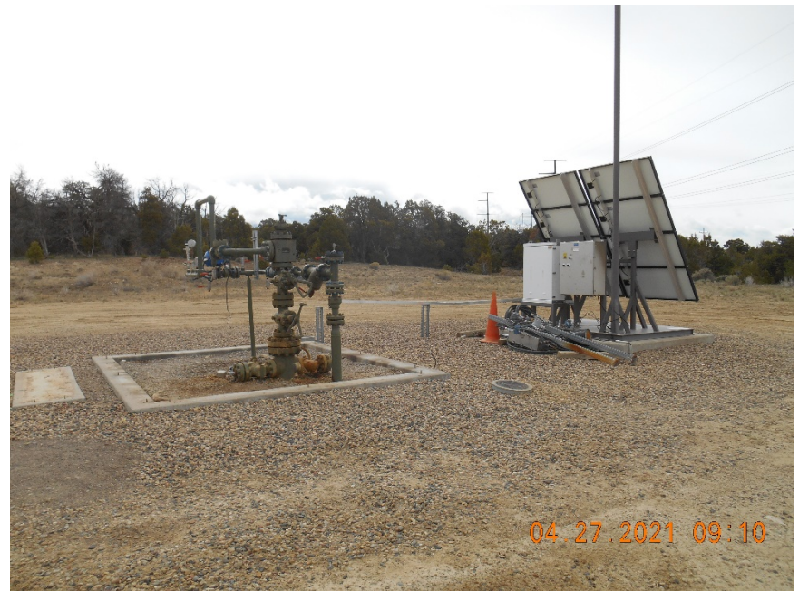
Injection wellhead with housing removed. Temporarily Abandoned
