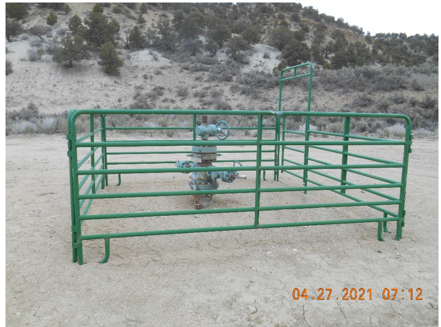
Injection wellhead with fence. Temporarily Abandoned
