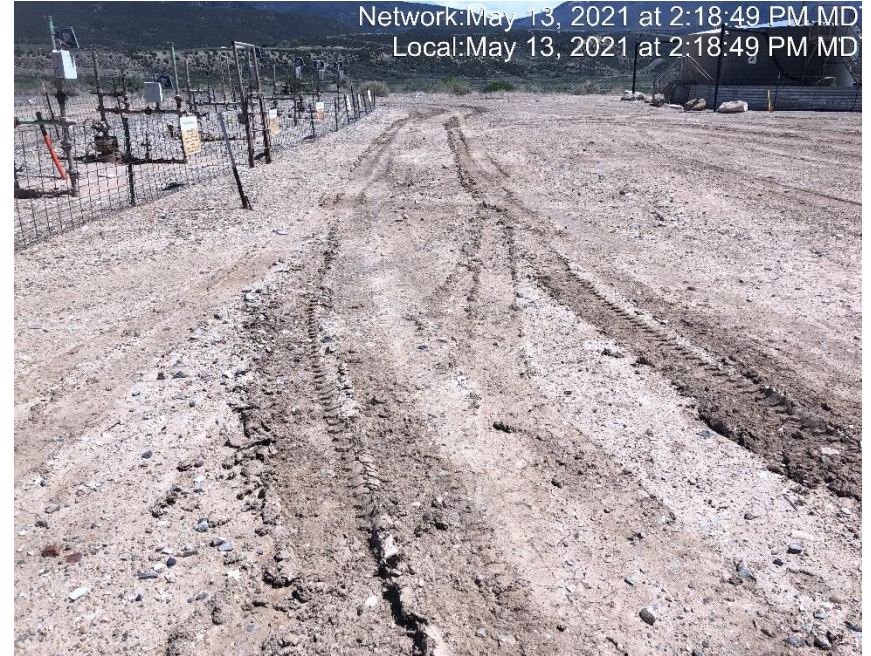
Photo #3806 Location lacks stabilization.
