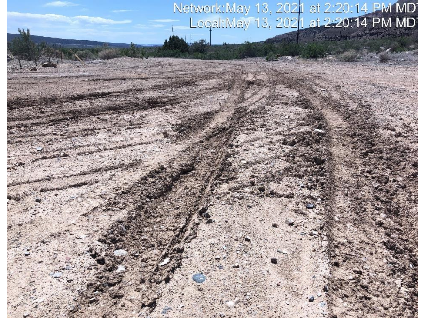
Photo #3808 No form of tracking BMP at entrance to location.
