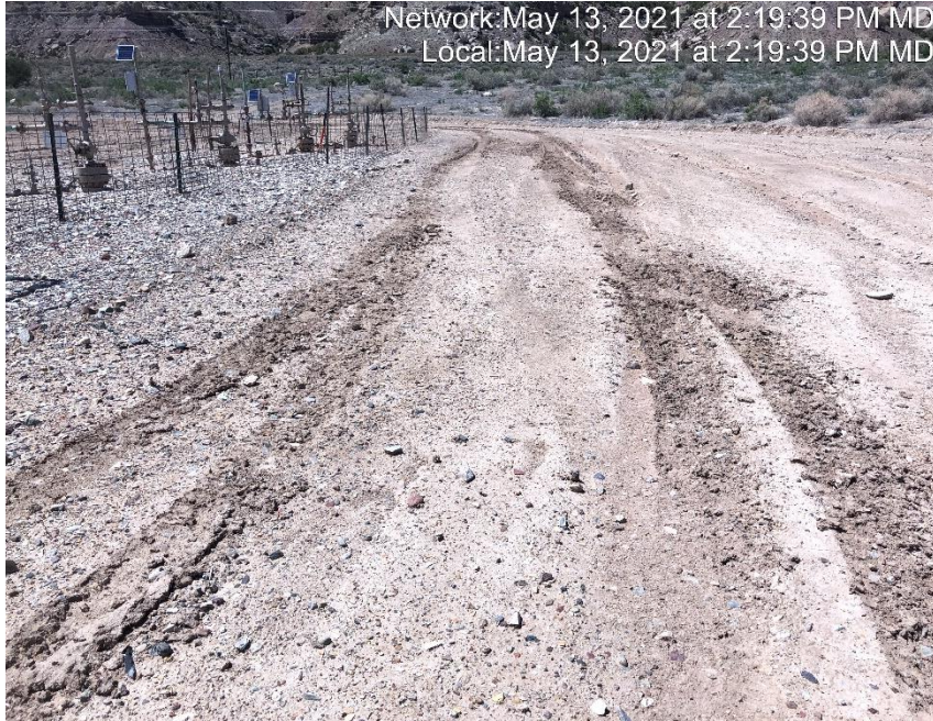
Photo #3807 Location lacks stabilization.
