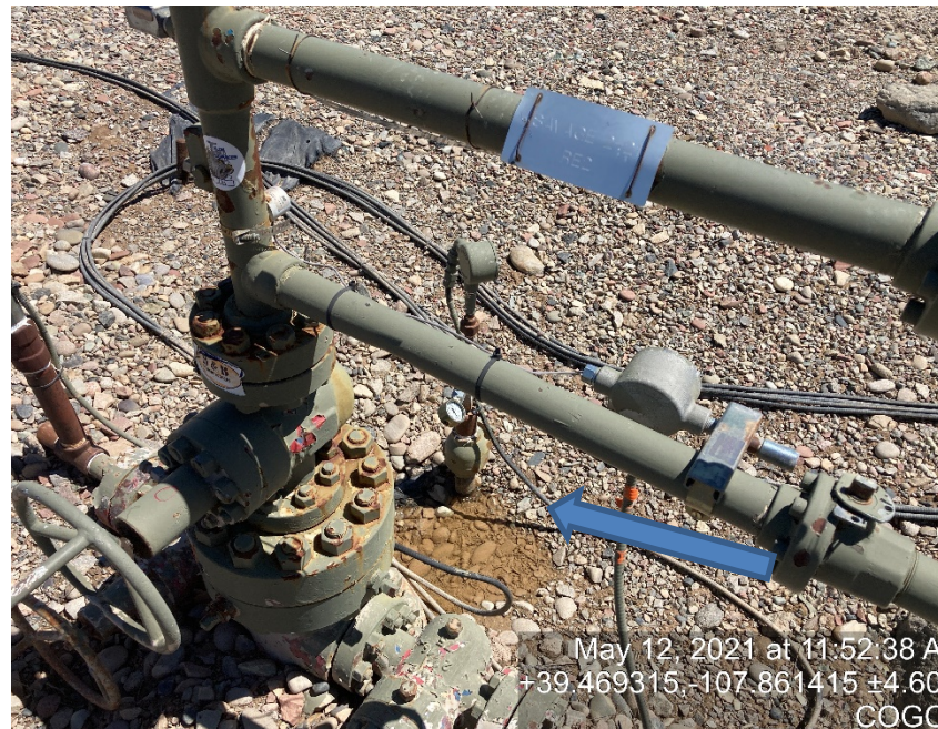
Braden head bubbling around piping
