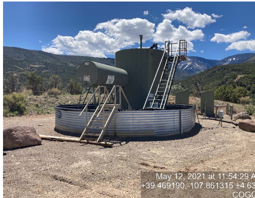
location/lack of battery signage
