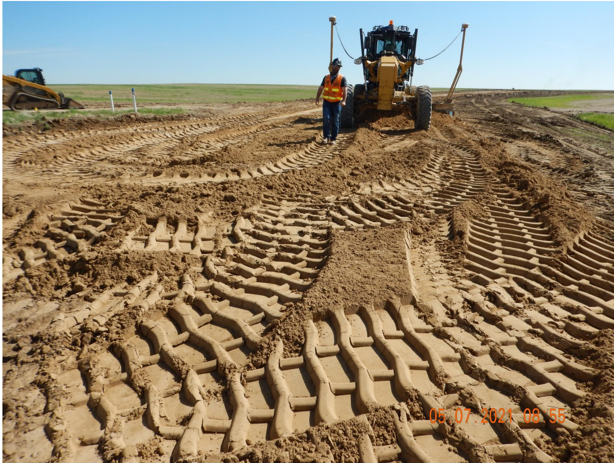
Photo 5. Photo taken from the entrance of location, facing East. Photo illustrates construction activities are underway along the access road.
