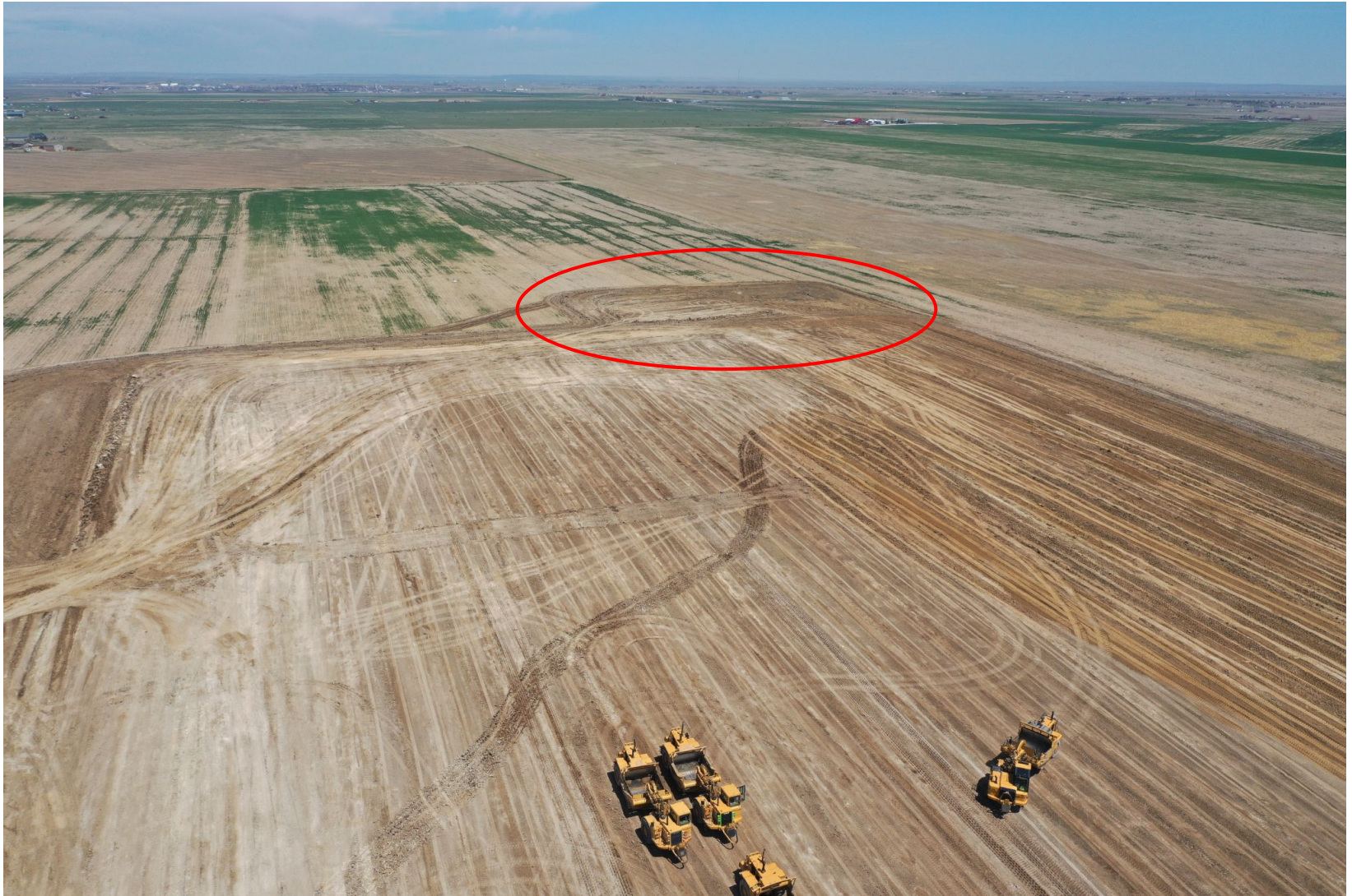
Photo 4. Drone aerial imagery taken during construction operations. Photo illustrates the detention pond.
