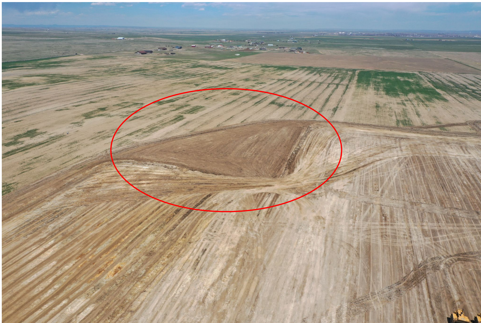
Photo 3. Drone aerial imagery taken during construction operations. Photo illustrates the topsoil stockpile.
