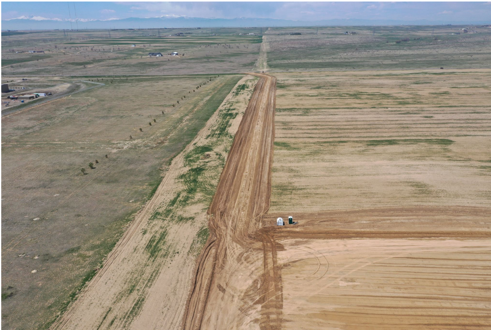
Photo 2. Drone aerial imagery taken during construction operations. Photo illustrates the access road.
