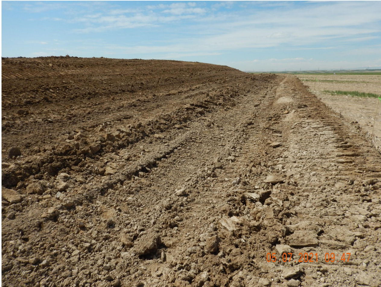
Photo 7. Photo taken from the western location, facing South. Photo illustrates a ditch BMP which is directed to a detention pond. Photo also illustrates the topsoil stockpile.
