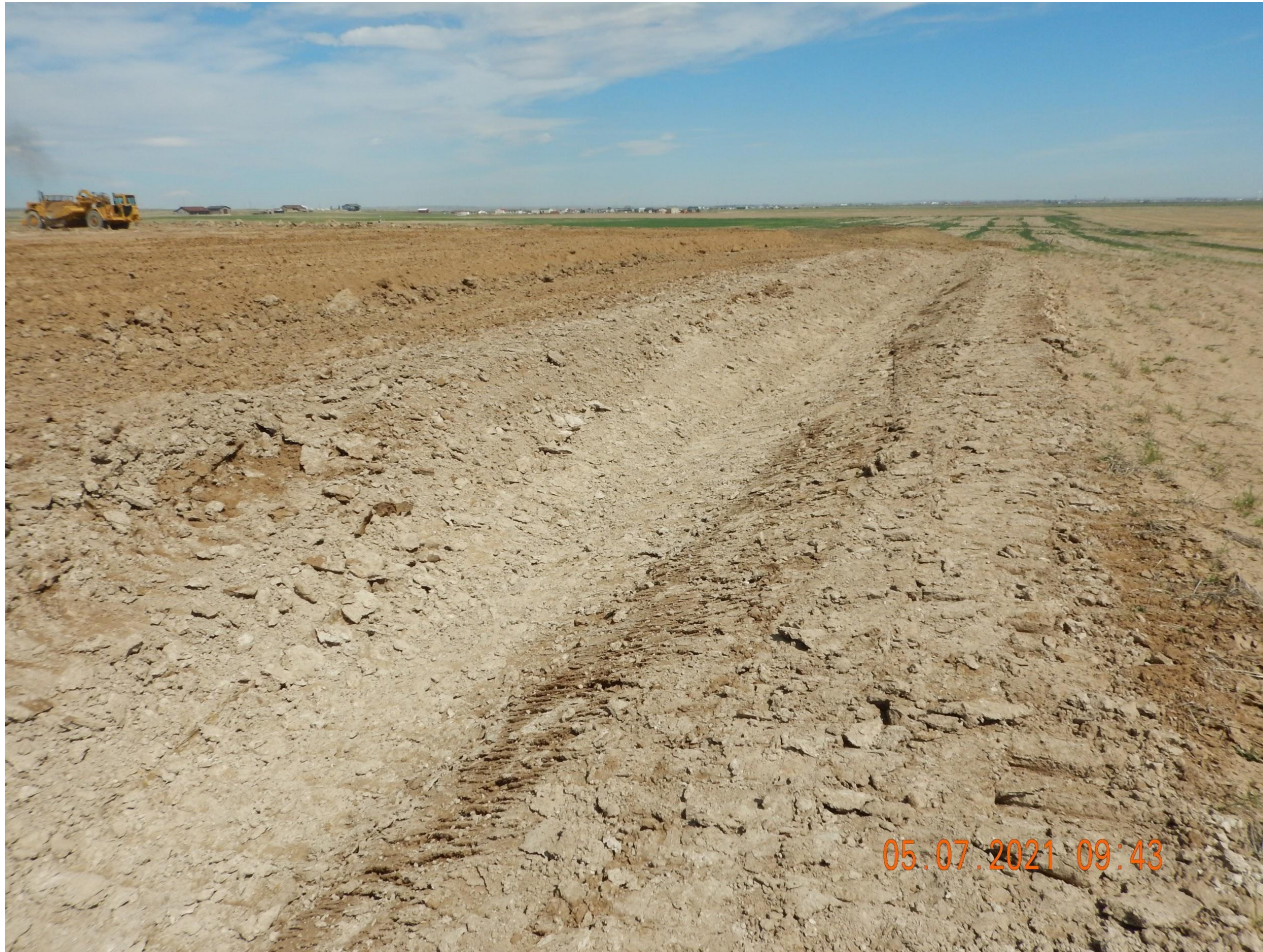
Photo 6. Photo taken from the eastern location, facing North. Photo illustrates a ditch BMP which is directed to a detention pond.
