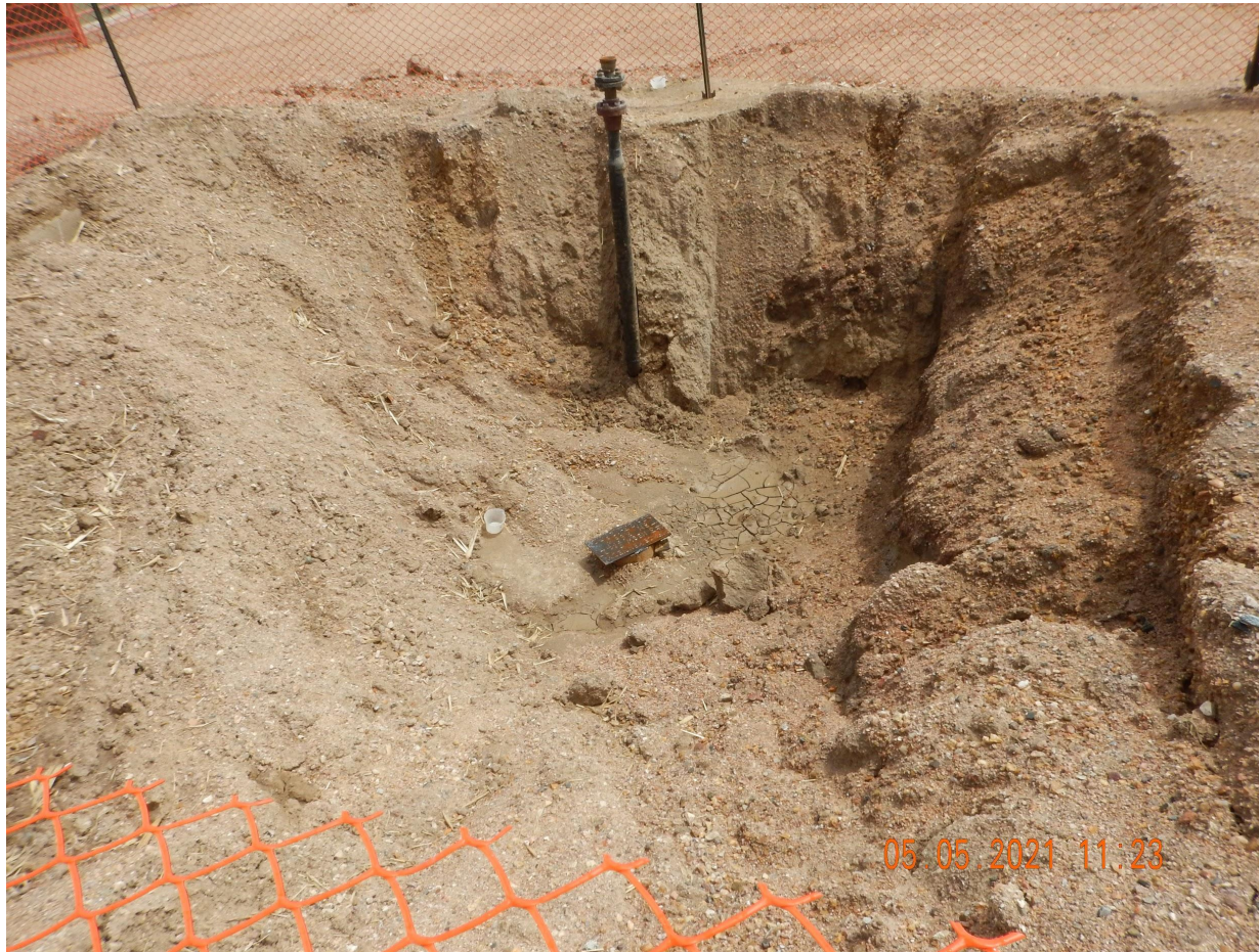
Photo 1. Photo taken from the location. Photo illustrates Operator is in process of plugging operations.
