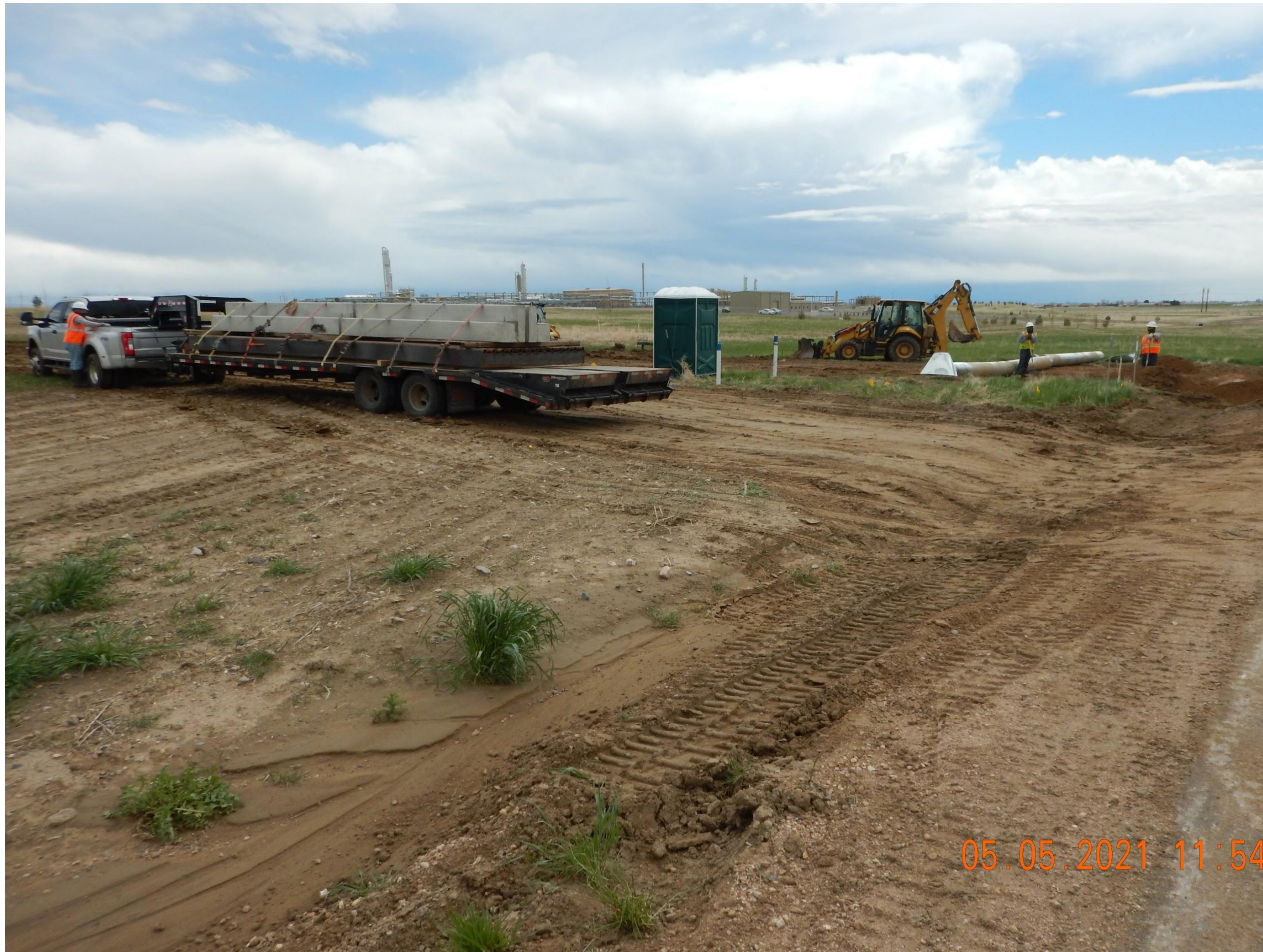
Photo 1. Photo taken from the entrance of location, facing South. Photo illustrates major construction activities have commenced.
