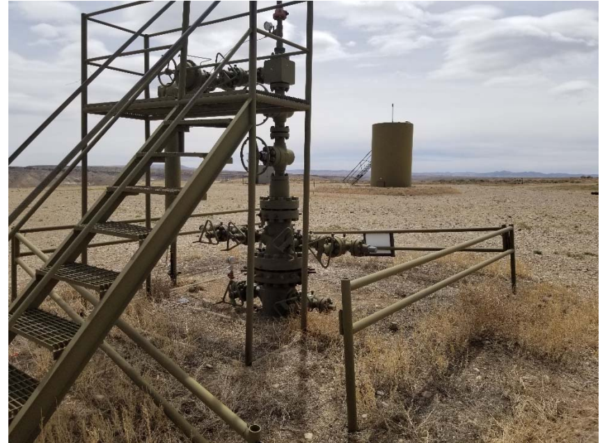
Photo 2. No bradenhead access apparent.
