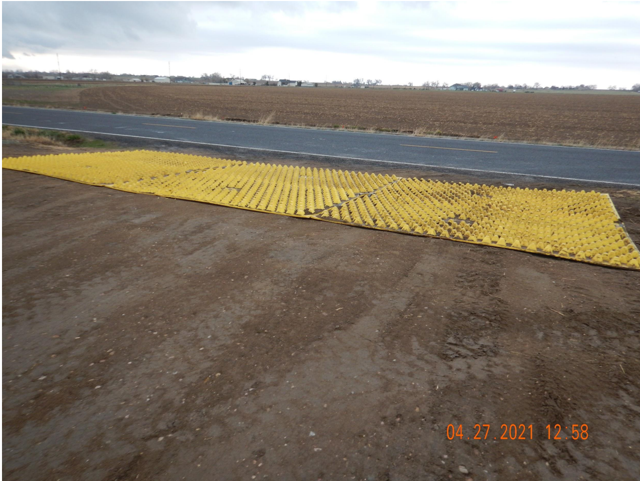
Photo 1. Photo taken from the entrance of location, facing East. Photo illustrates Operator has installed a vehicle tracking device BMP. At the time of this inspection, no vehicle track out issues were observed.
