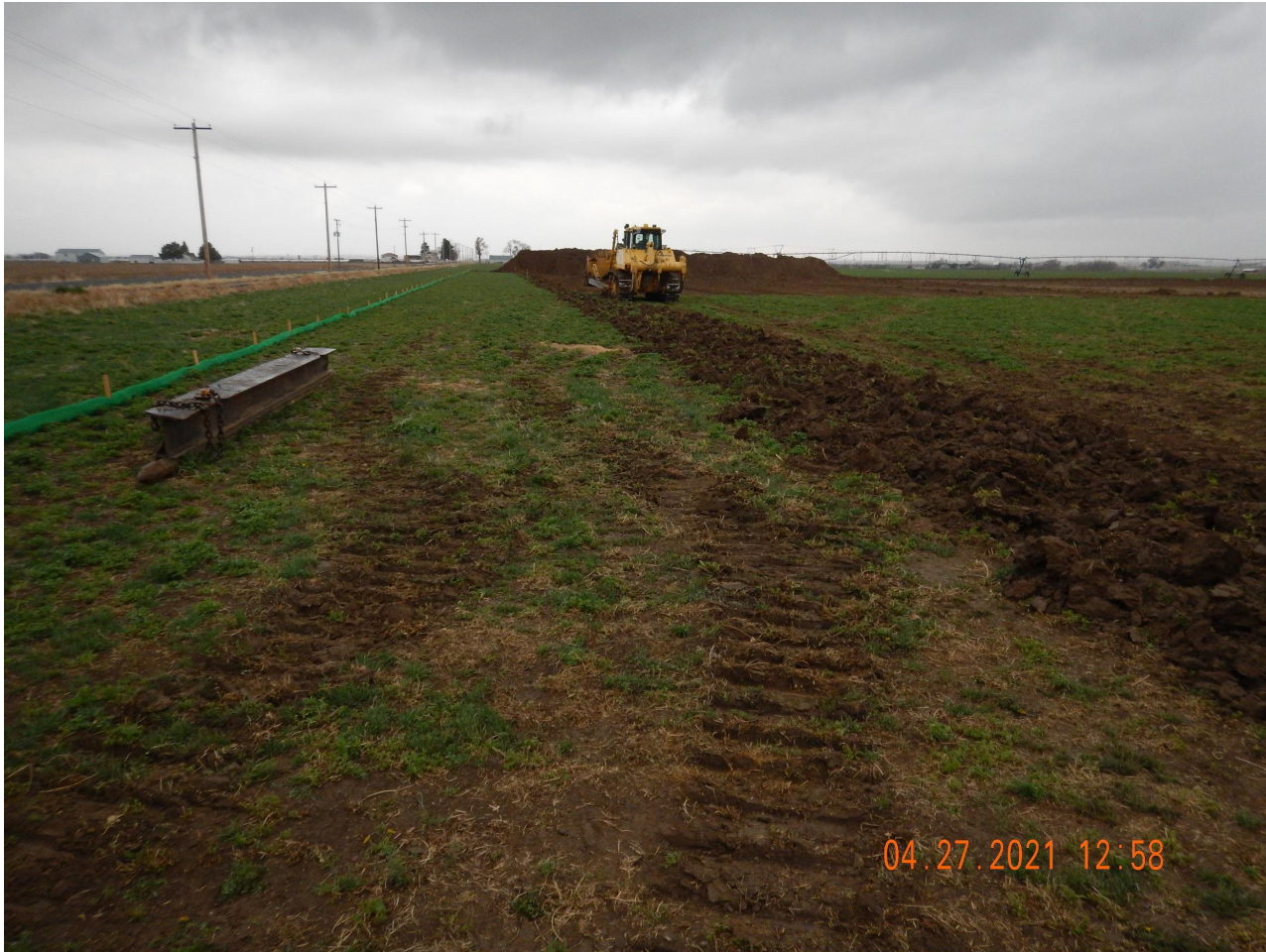
Photo 2. Photo taken from the northeastern location, facing South. Photo illustrates Operator has installed surface roughening and filter wattle BMPs around the entire perimeter of location. Topsoil is being salvaged and stored along the southern and western perimeter of the location.
