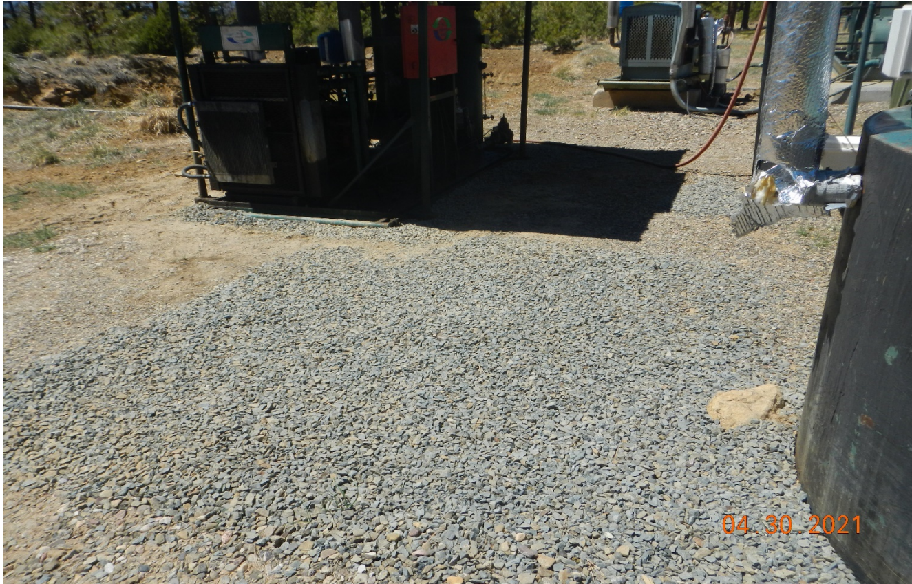
Photo 3. The stained soil near the engine skid has been cleaned up.
